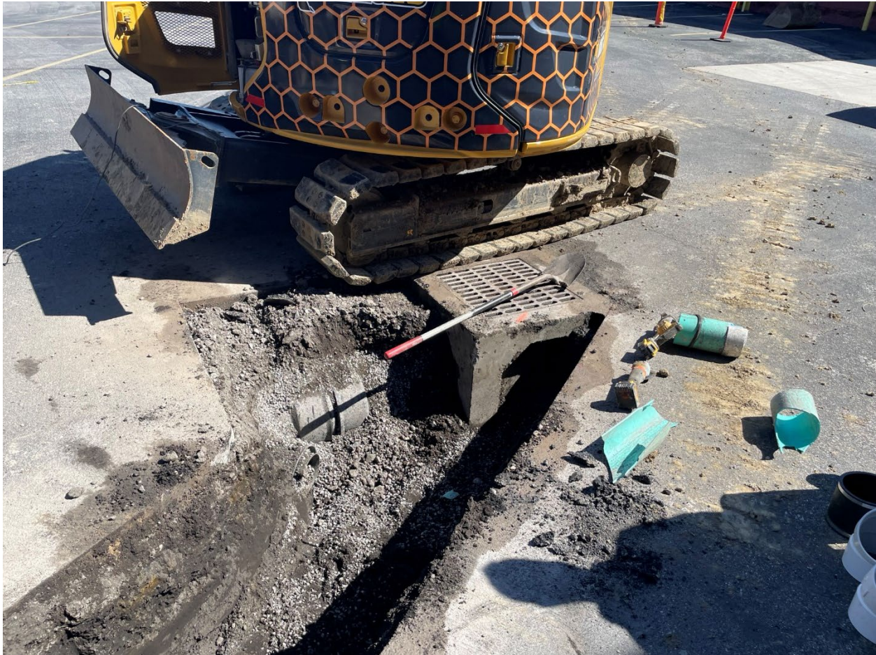
View of trench with stormwater catch basin that a 4inch line will be tied into and broken 6-inch HDPE line pending connection repair which was to be performed by Dirtworks on this date.
