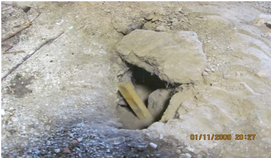
3. Hole in southern most bay floor
