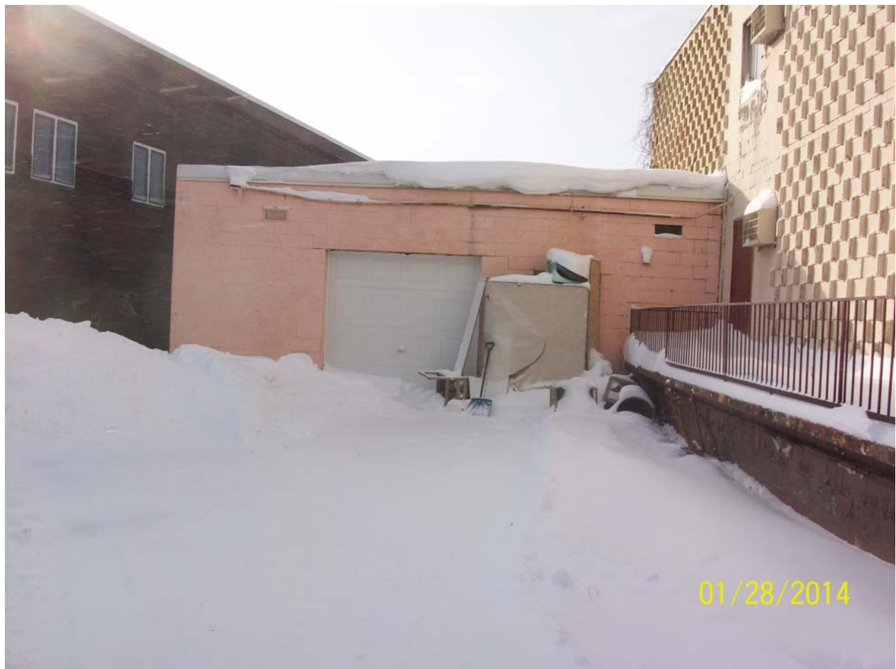
Photo 6: Garage used for storage attached on the east side of the south motel building.
