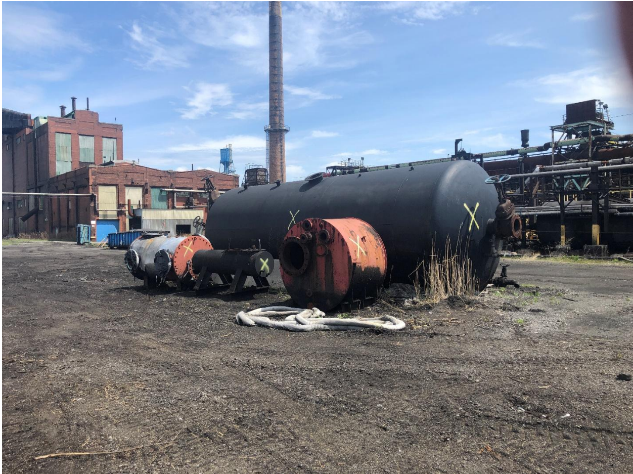
Photograph No. 3: ST27 was onsite and never installed (large black horizontal cylinder). The three additional smaller vessels in the photograph were gas venting vessels associated with the Boiler House and the flares that never contained liquids. They were also removed, cleaned, and recycled.
