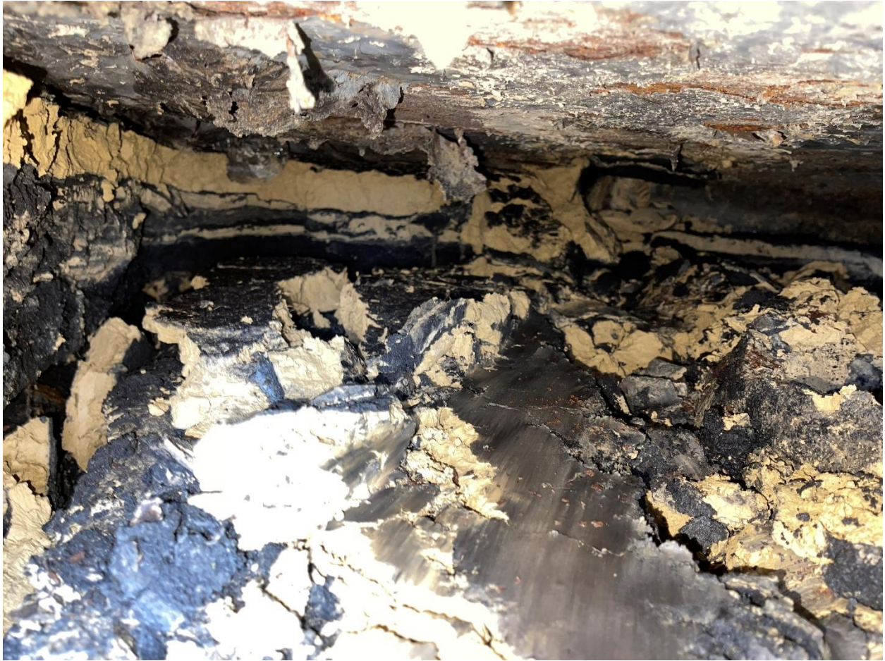
Photograph 3: Lid Seal Material Below Secondary Containment of ST06.
