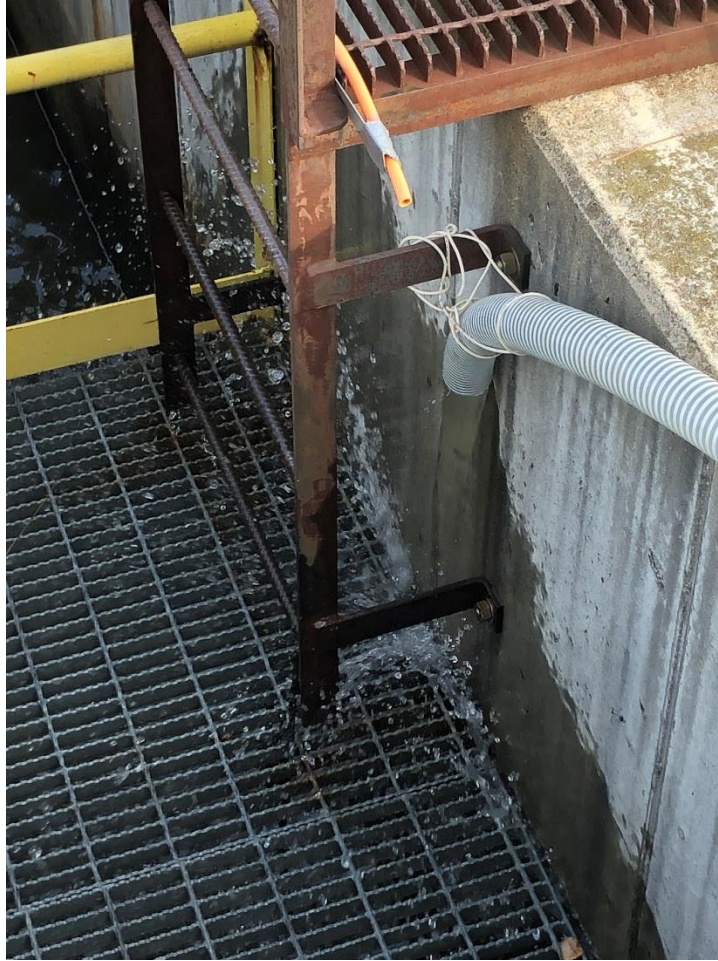
Filter Discharge – Upstream of Flume and Flow Meter December 2020
