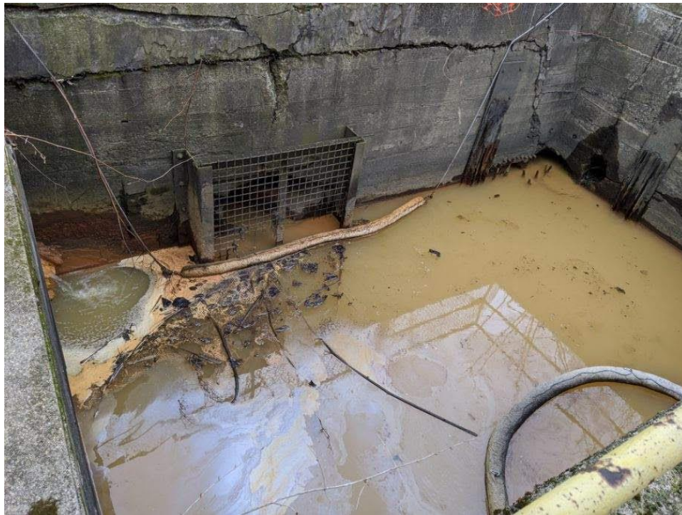
Mansion Sump at Time of Transfer to Riverview, Prior to Cleaning January 2020
