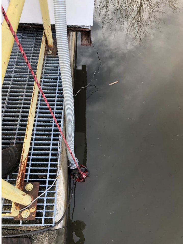
Pump Location December 2020
