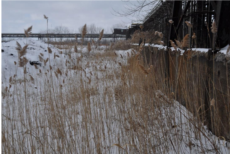
Photograph No. 2 Depression next to Coal Breaker Building (Looking West)
