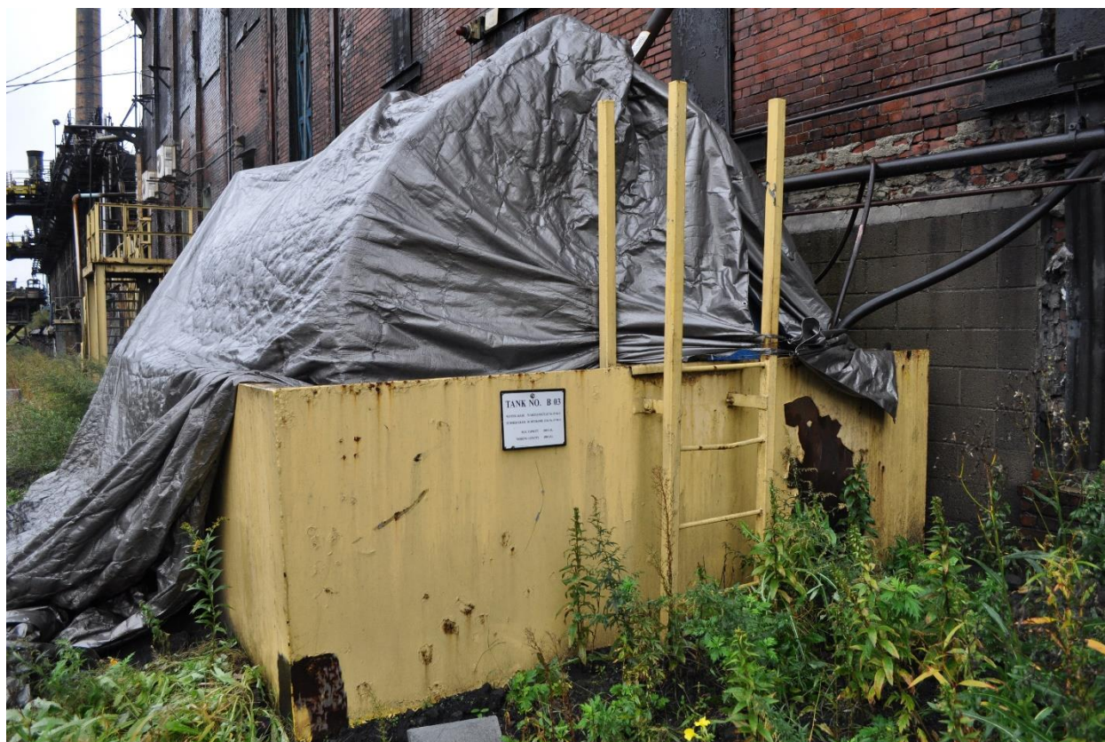
Secondary Containment for Lid Seal Tank
