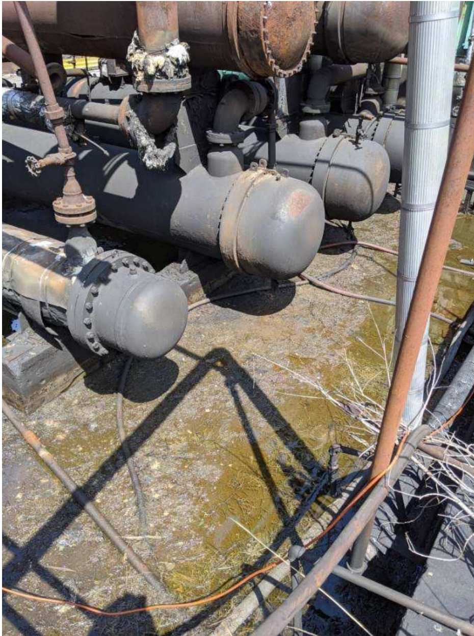
Photograph No. 4 – Chillers in Light Oil Area Secondary Containment (Note Rupture)
