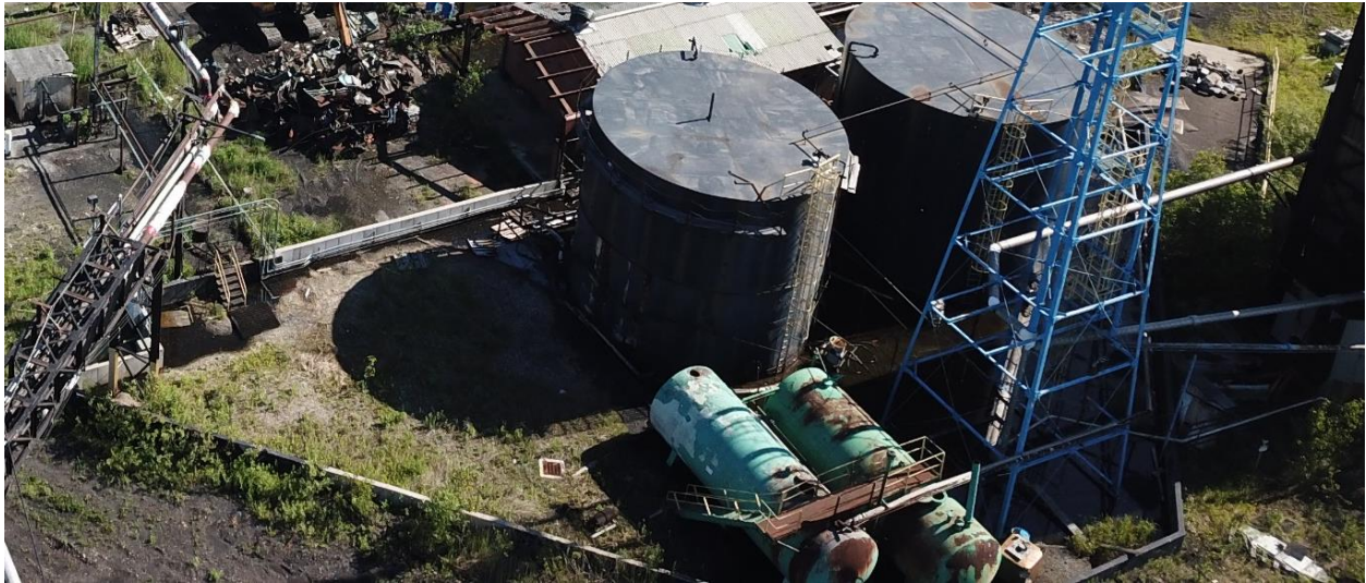
Weak Ammonia Tank Secondary Containment
