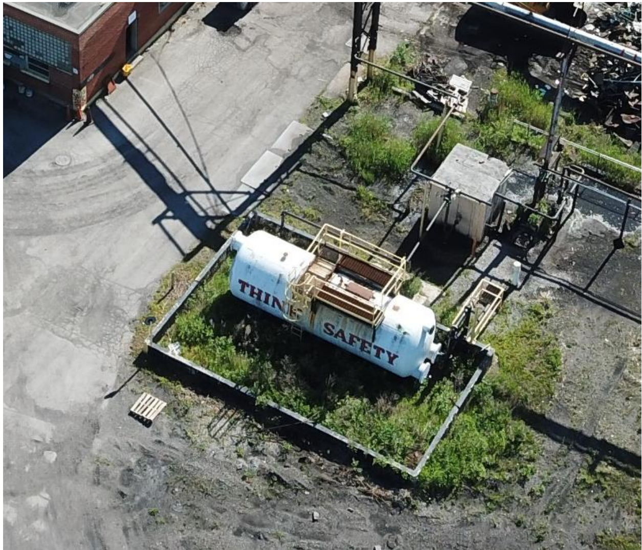
OWS Secondary Containment
