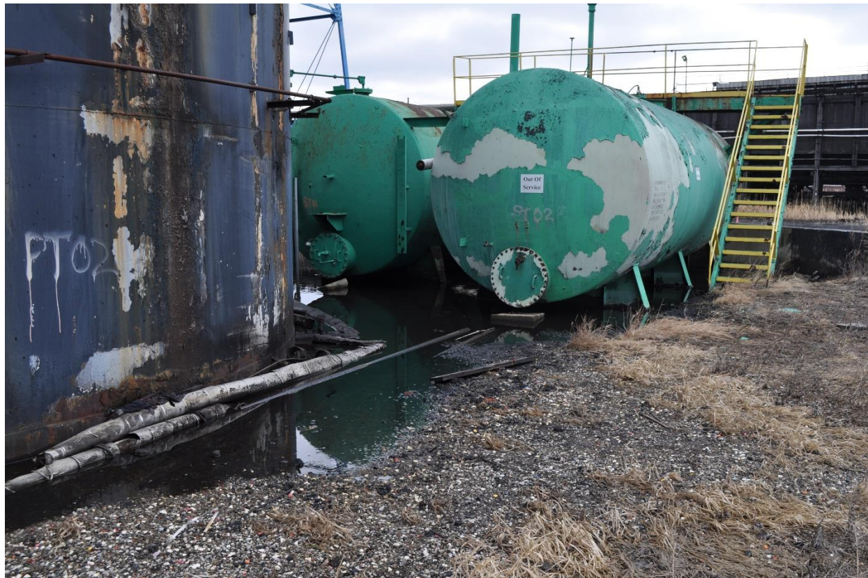
Photograph No. 6 - Secondary Containment Slab Appears to have been placed around the Weak Ammonia Tank Foundations (PT02 and PT03)
