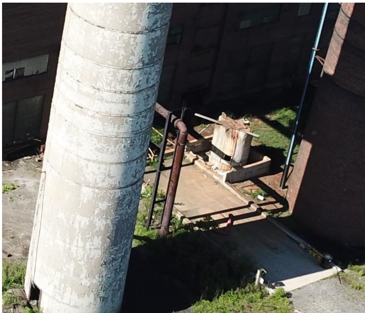
Caustic Tank Secondary Containment
