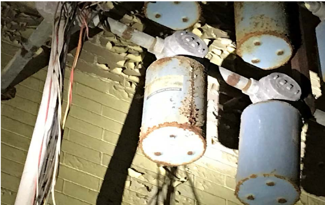
PHOTO #5- Photograph of ballast for high discharge lights.
