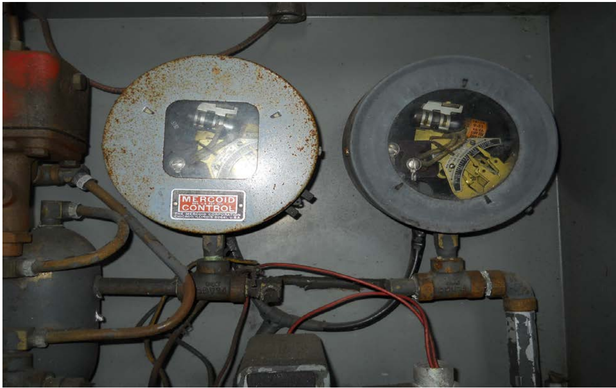
PHOTO #9- Photograph of the mercury-containing pressure control swithes.
