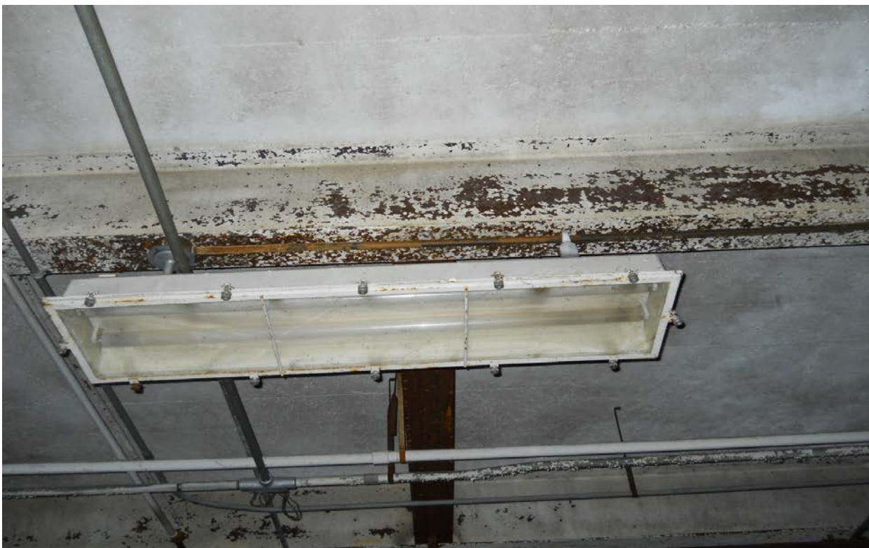
PHOTO #6- Photograph of fluorescent light fixtures (typical). Note, the light cover gaskets are asbestos-containing.
