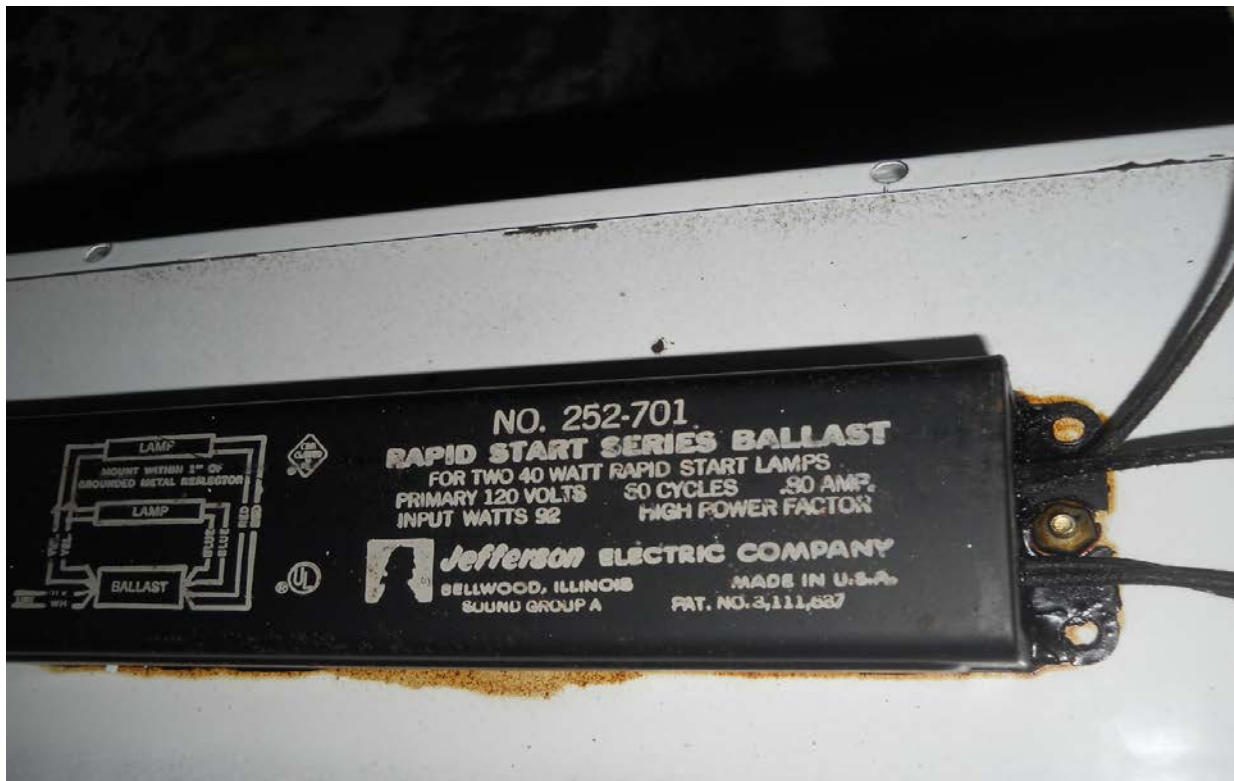
PHOTO #8- Photograph of fluorescent light fixture ballast (typical).
