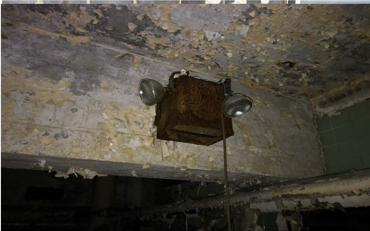
PHOTO #1- Photograph of the emergency exit lights (typical) with back-up battery.
