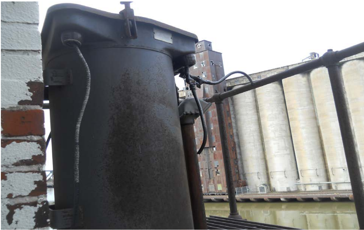
PHOTO #3- Photograph of exterior transformer on Building 1.
