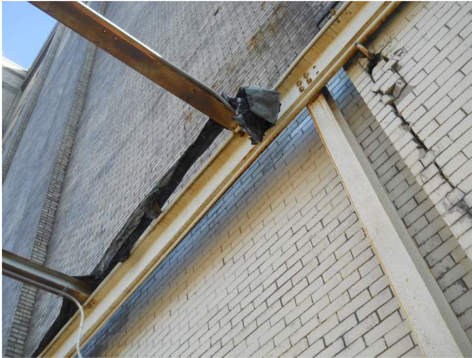
Photo 1 – View of lead-based paint coated exterior structural steel at Building 1.
