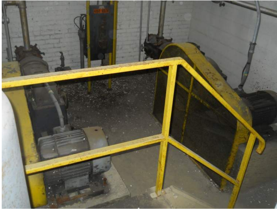
Photo 5 – View of a lead-based paint coated hand rail on the second floor of Building 1.
