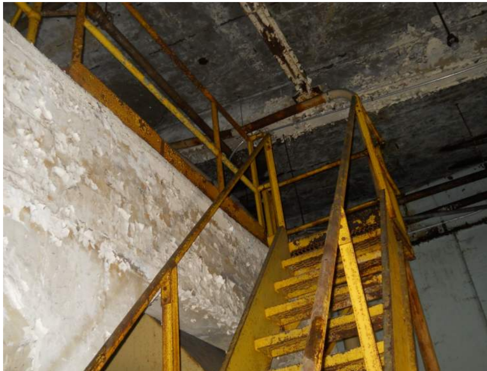
Photo 3 – View of lead-based paint coated staircase on the eighth floor of Building 2.
