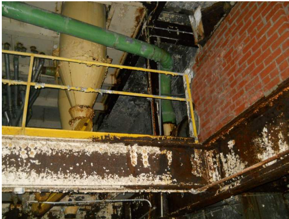
Photo 7 – View of lead-based paint coated hand rails and structural beams in Building 1.
