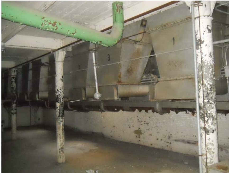
Photo 6 – View of lead-based paint coated columns in Building 1.
