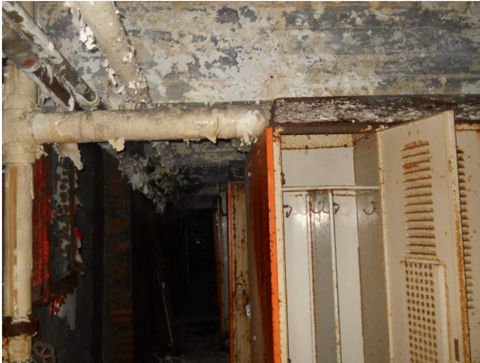
Photo 2 – View of lead-based paint coated lockers on the second floor of Building 2.
