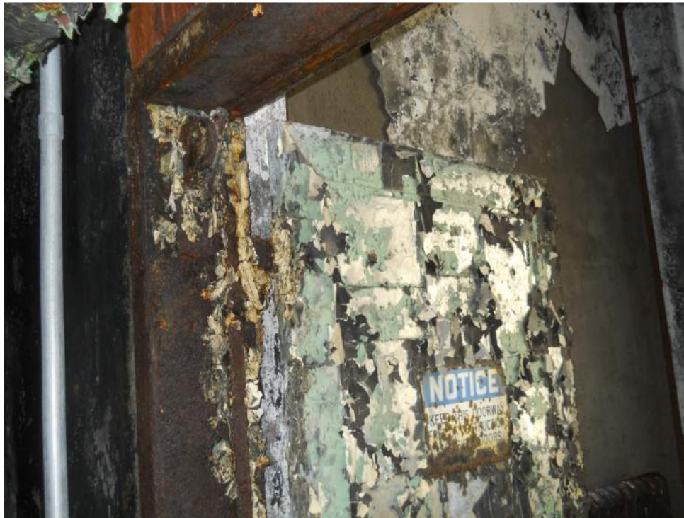
Photo 8 – View of lead-based paint coated blast door and frame in Building 2.
