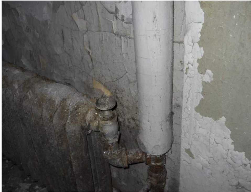
Photo 3 – View of a lead-based paint coated radiator in Building 2.
