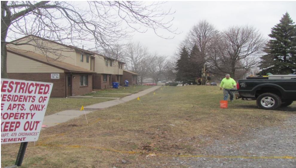
17. Location of Borehole BH-6 (Top of Berm) eastern side of property along Michigan Ave. from south facing north
