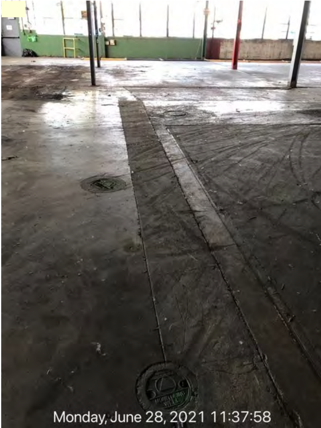
Photo 7: Building Slab Cover System with Varnish Pit Monitoring Well (typ)
