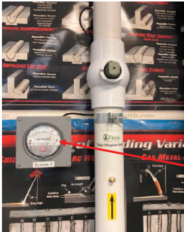
Figure 3.01F: Example of Monitoring Panel
