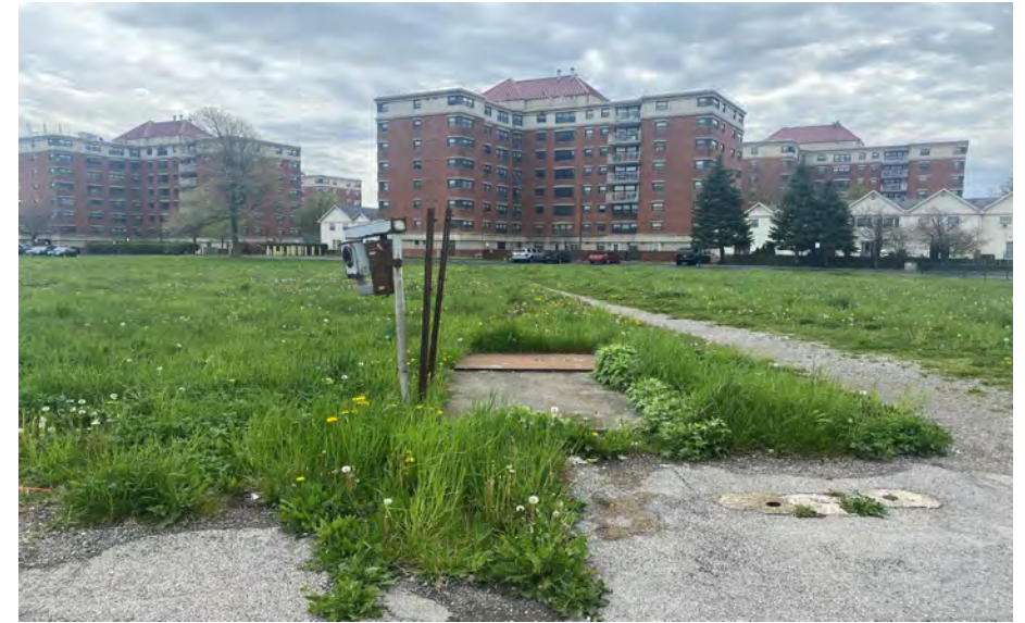
18. Old meter post on cement pad and metal plate – southwest side (says Buffalo Water Authority)
