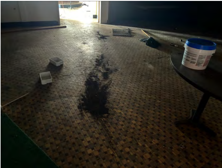
39. Floor staining in northeastern room of 680 Amherst Street.
