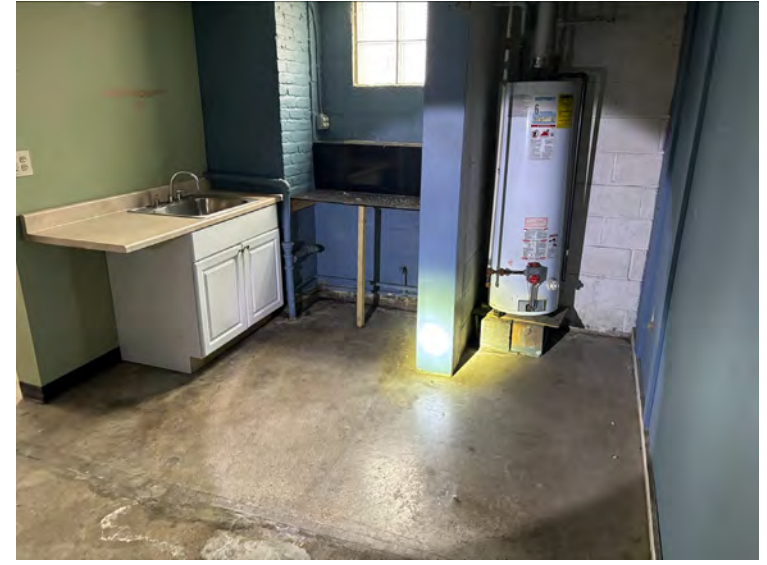
34. View of hot water heater on southern portion of 1628 Elmwood Avenue.
