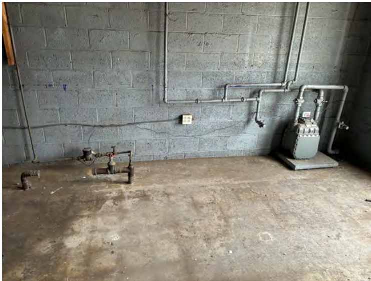
31. Utilities on eastern portion of 1628 Elmwood Avenue.
