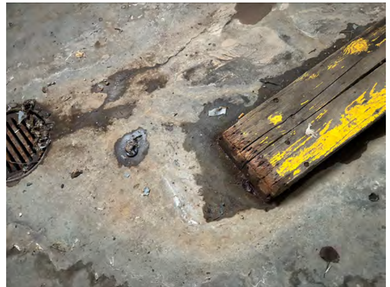
22. Floor drain and floor staining on northside interior of 155 Marion Street.
