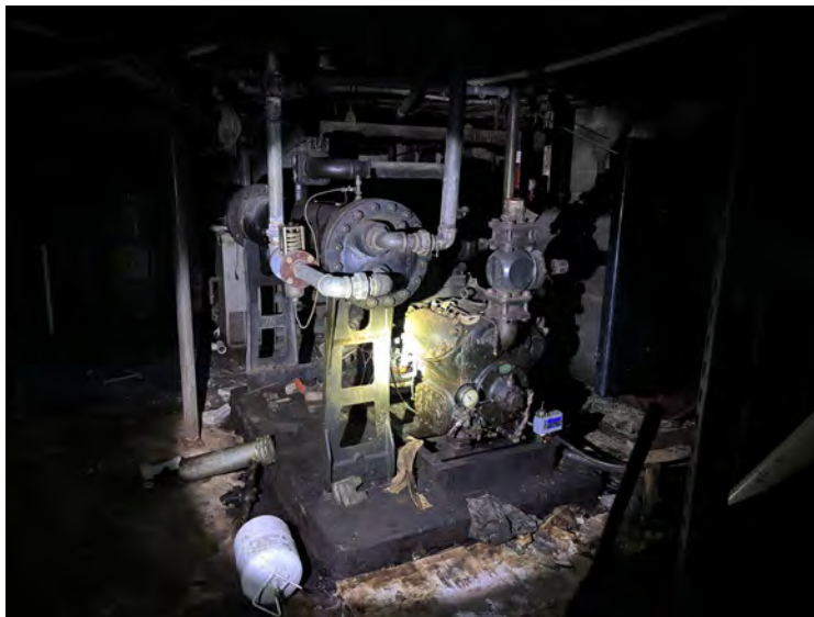
47. Utilities in basement of 680 Amherst Street.
