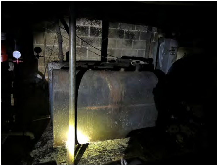
45. Tank in basement of 680 Amherst Street.
