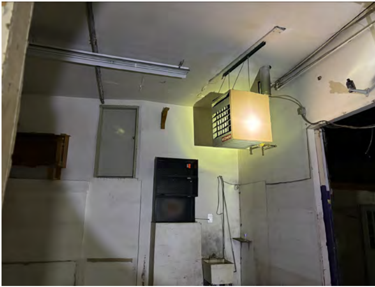
33. View of heater on southern portion of 1628 Elmwood Avenue
