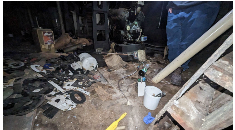
38. View of SS-2 location in basement
