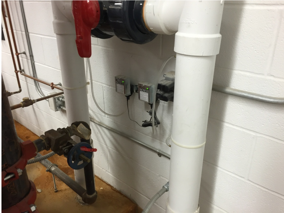
Photograph No. 5 – Sub-slab Depressurization System in basement, depicting alarms and stack discharge piping.
