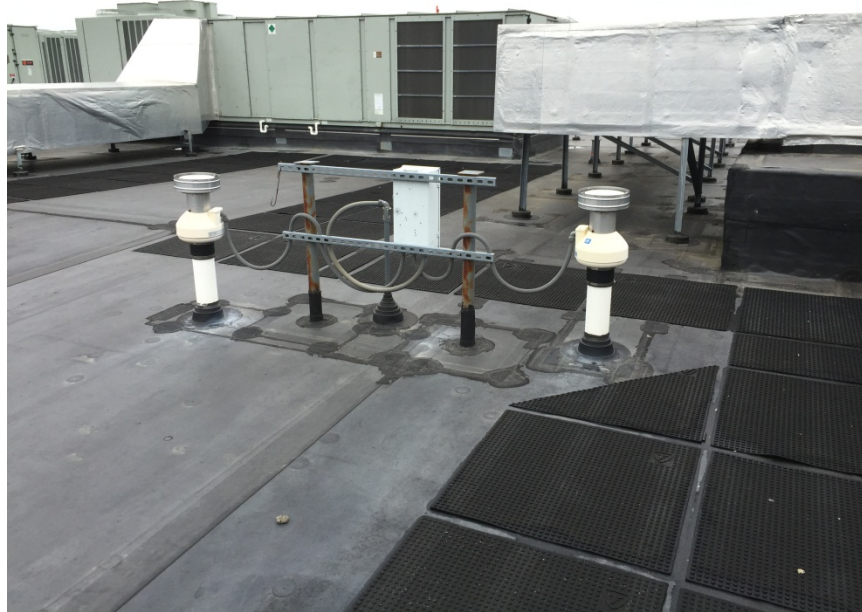
Photograph No. 6 – Sub-slab Depressurization System discharge vents and blowers and power control for discharge vents.
