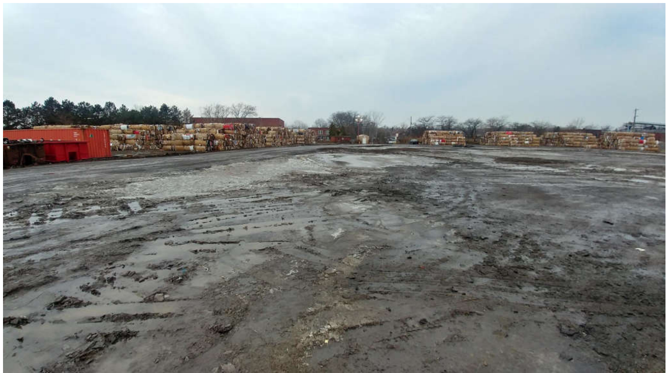
Photo #2: Ponding near high-traffic areas.
