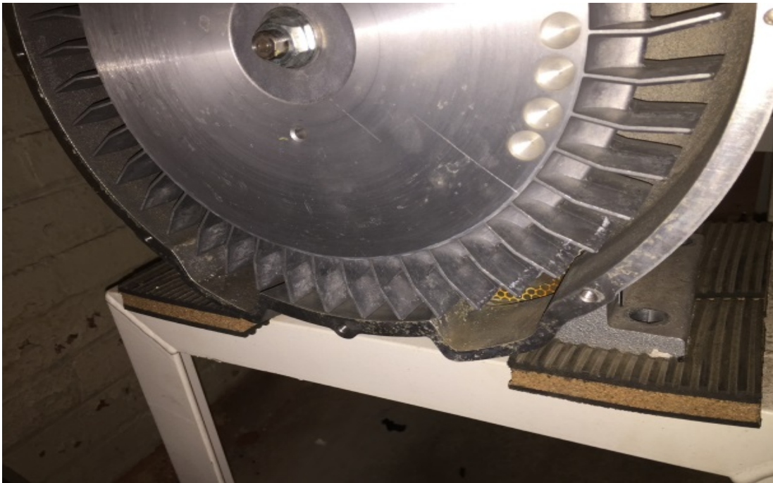
Photo #2: SSDS Blower 7A-2 – Impeller (minor oxidation observed)
