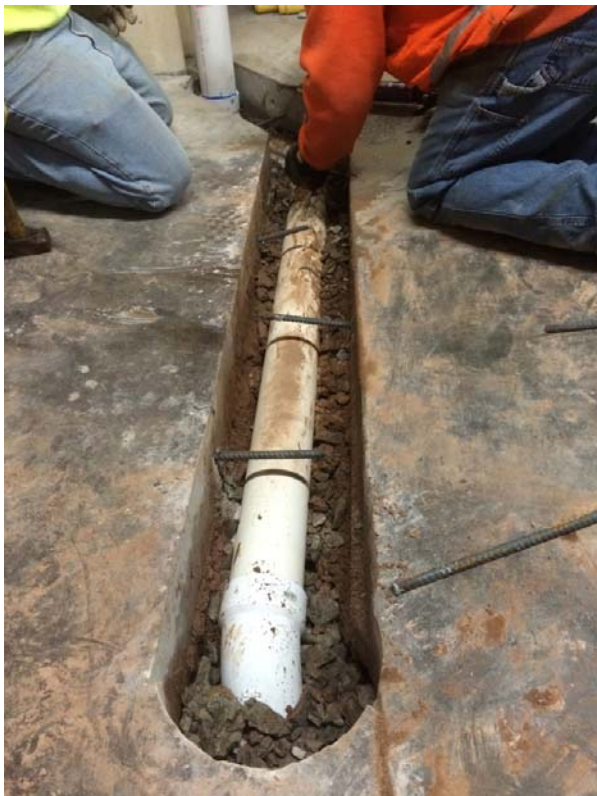
New sub grade SSD piping from suction pit to stub-up at column.
