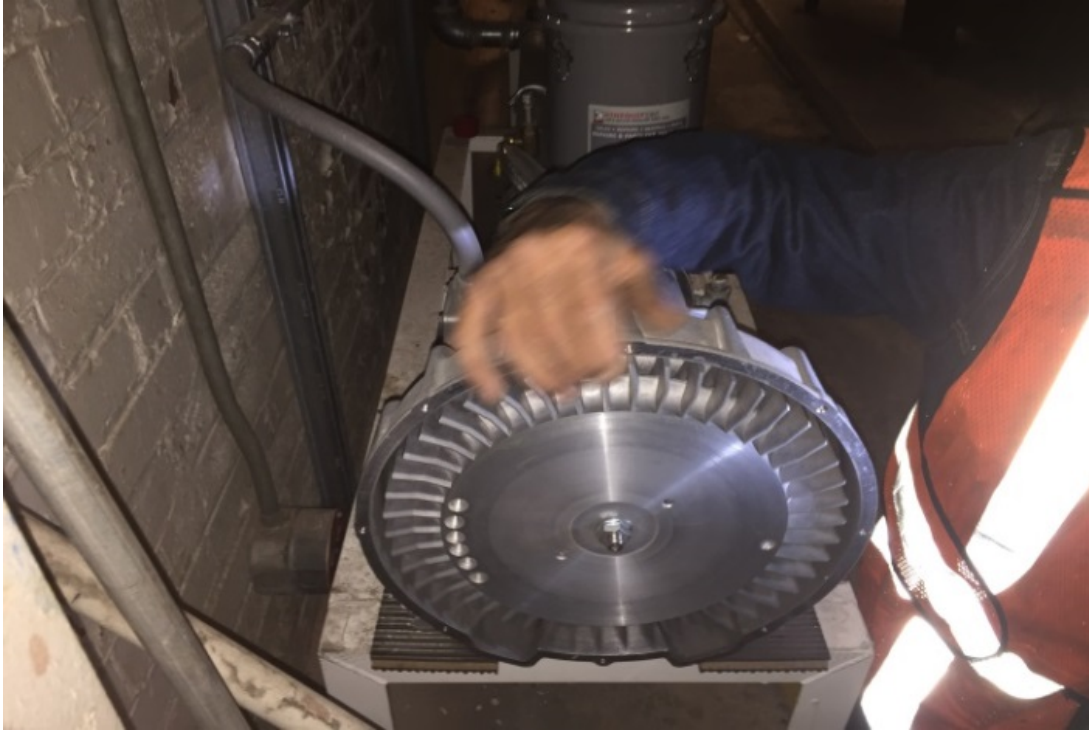
Photo #1: SSDS Blower 7A-1 - Impeller
