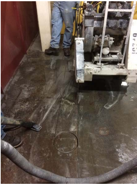
After concrete coring at new suction pit location and cutting for placement for sub grade piping.
