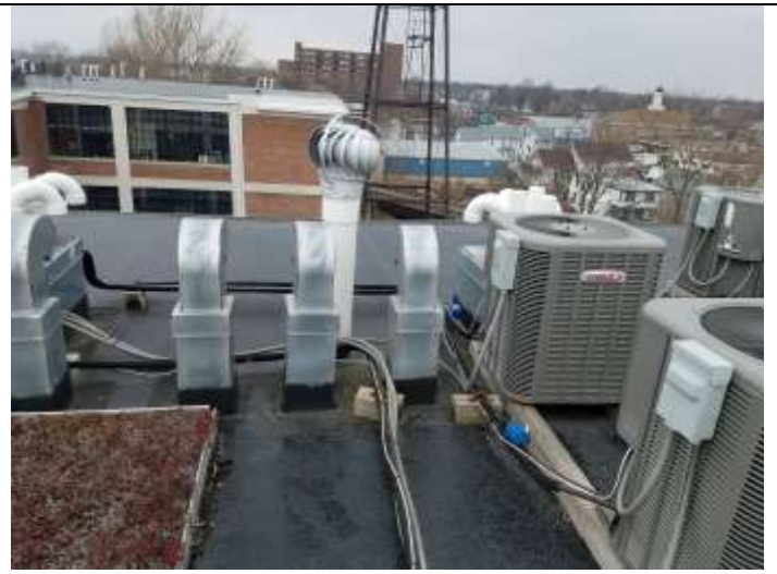
SSDS Roof Vent
