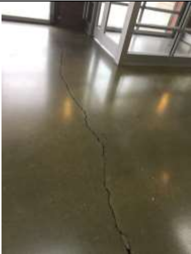
Floor crack in lobby
