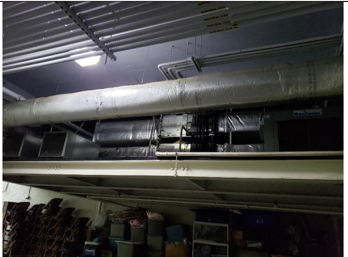
HVAC system associated with Remington Tavern
