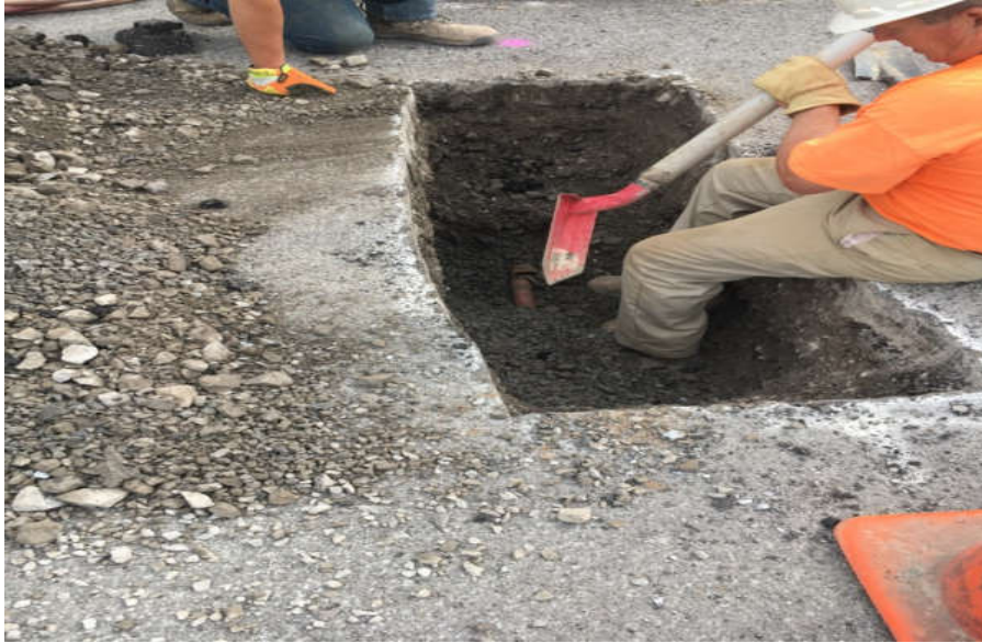
Photo 3: Damaged communications line uncovered through excavation.
