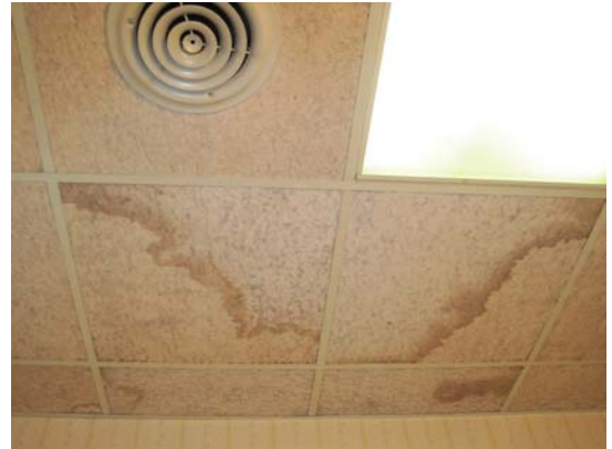
Minimal water damage on ceiling tiles within Site building
