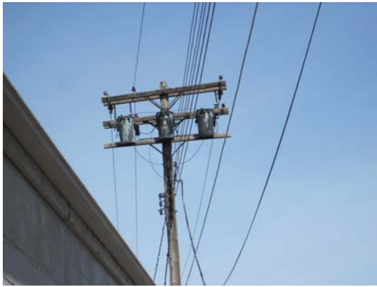
Three pole mounted transformer on eastern portion of Site
