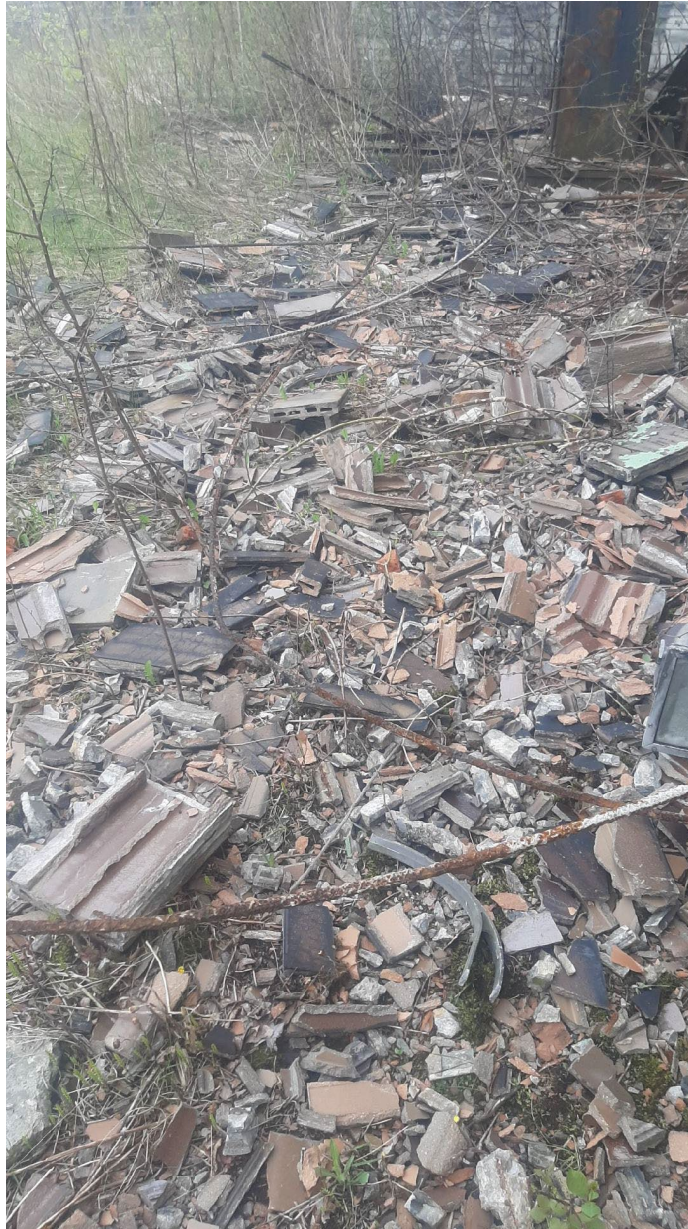
Figure 2. Fall Debris (tiles) from Former Coal Storage Silo
