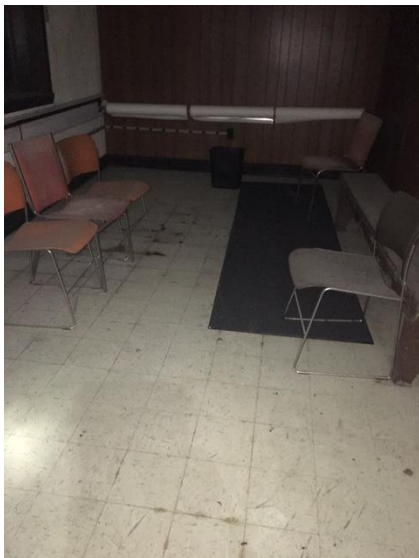
Photo 3: White Speckled 9" Asbestos-Containing Floor Tile in Rear Office Area on 1 ST Floor.
