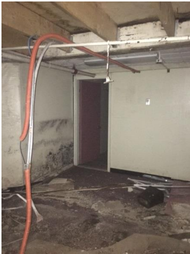
Photo 2: Visible Mold Growth on Drywall
