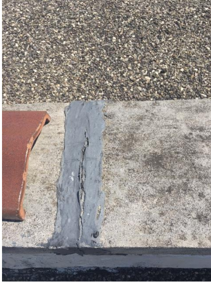
Photo 9: Black Asbestos-Containing Tar on Exposed Coping of Parapet Wall.
