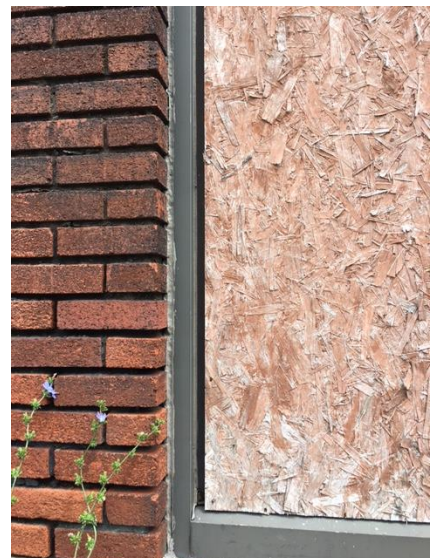
Photo 4: Gray Asbestos- Containing Window Caulk on West Side Exterior Window.
