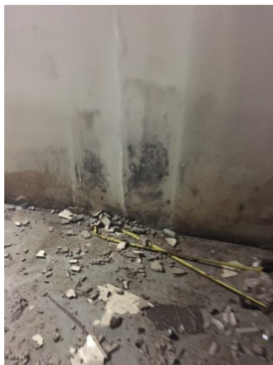
Photo 3: Visible Mold Growth on Drywall
