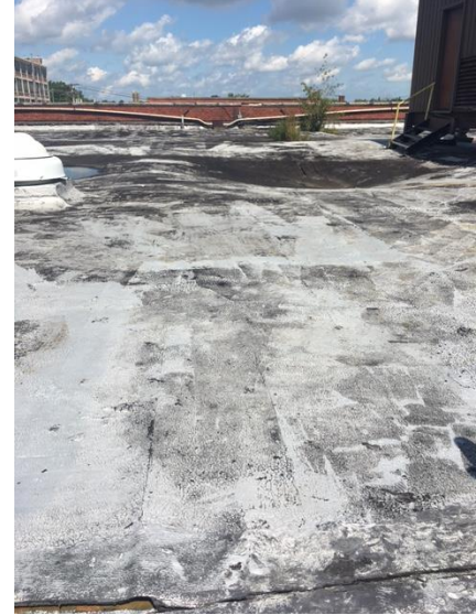
Photo 10: Black/Silver Asbestos-Containing Roof on 1925 Roof.
