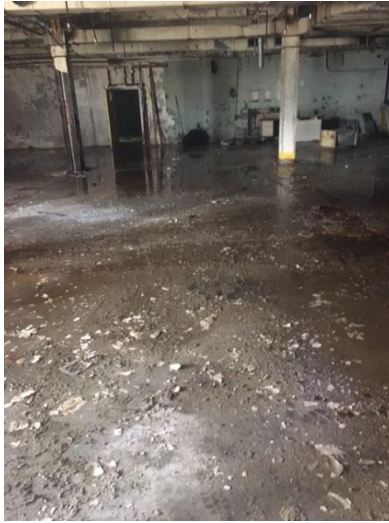
Photo 1: Severe Water Infiltration in E-Room Area
