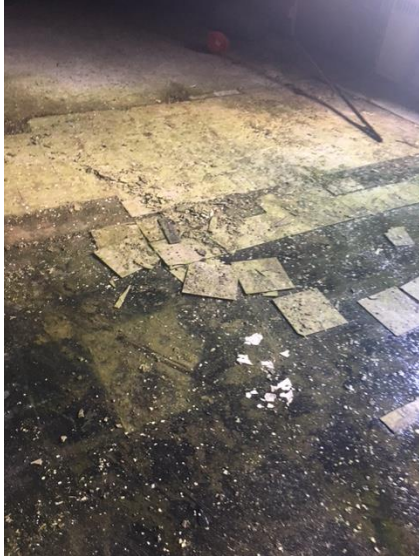
Photo 5: Tan 9" Asbestos-Containing Floor Tile in E-Room. (Incidental Disturbance)
