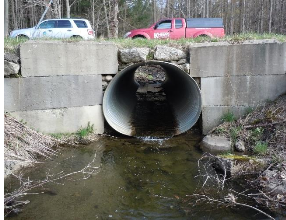
Image 6: Surveyed Bloomer Road stream gauging point at the top center (small hole in pipe) of the south side of the 60" culvert pipe
