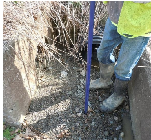
Image 4: Surveying ditch on southside Route 430. (Discharge pipe on shown on left transfers flow from north side of street to the south side)
