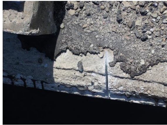
Image 8: Surveyed saw cut on bridge along Morris Street.
