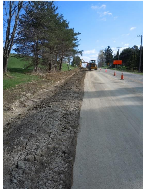
Image 2: Excavation of concrete lined ditch along north side of Route 430 (northeast direction)
