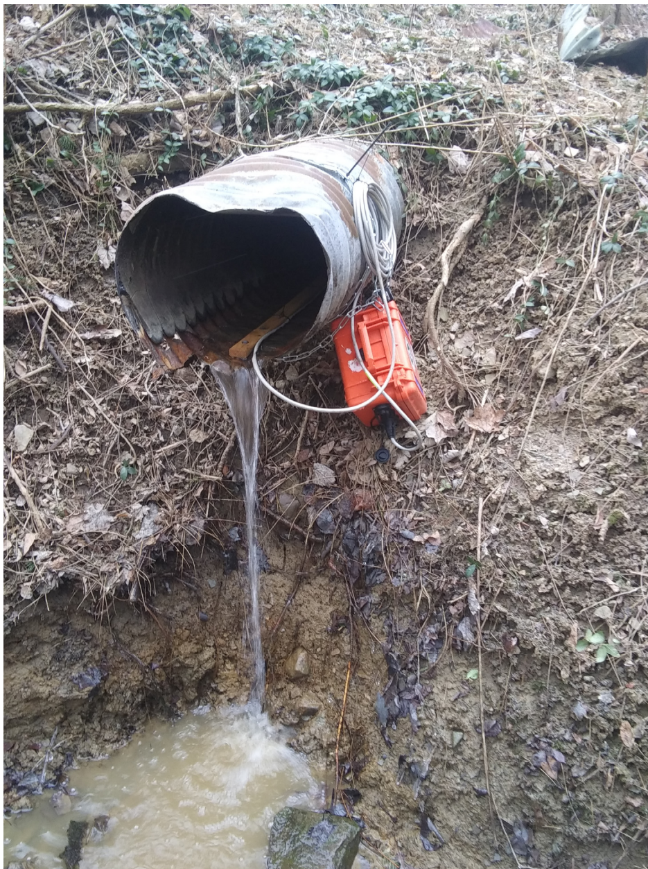
2/22/2023 9:14 AM - View to the north. Reduced discharge flow volume.
