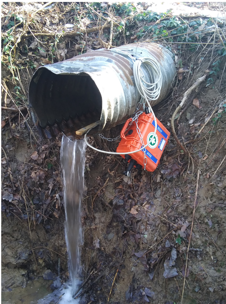
2/8/2023 10:05 AM - View to the north. Discharge pipe and initial datalogger deployment in the standard configuration during monitoring.
