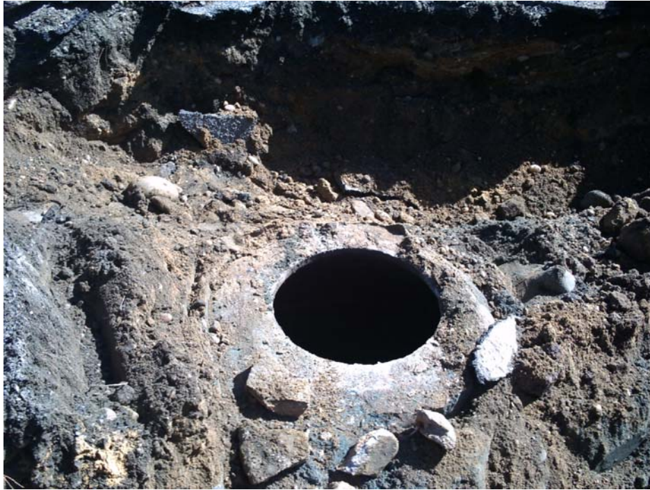
Drywell encountered two feet below grade.
