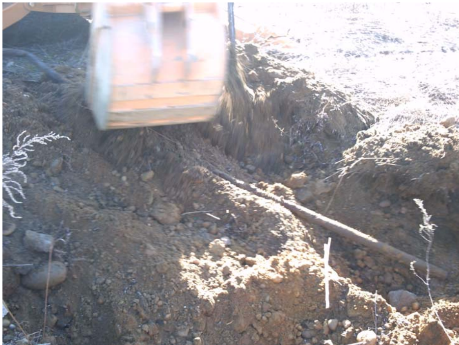
Two inch diameter steel pipes found at two feet below grade. These pipes are most likely associated with the USTs removed from the site.
