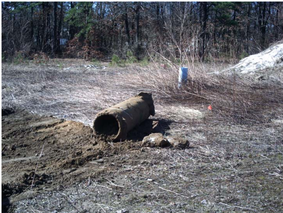
A two foot diameter concrete pipe was found at two feet below grade.
