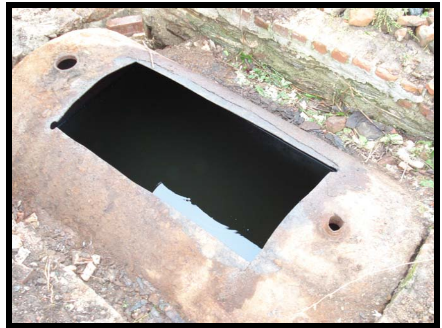
Photo 32 - View of Product in UST B
