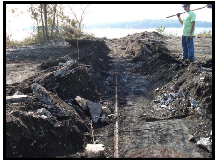
Photo 20 – View of UST A Piping Looking South
