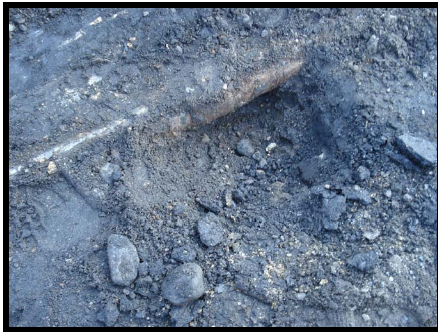
Photo 23 – Typical UST A Piping Joint
