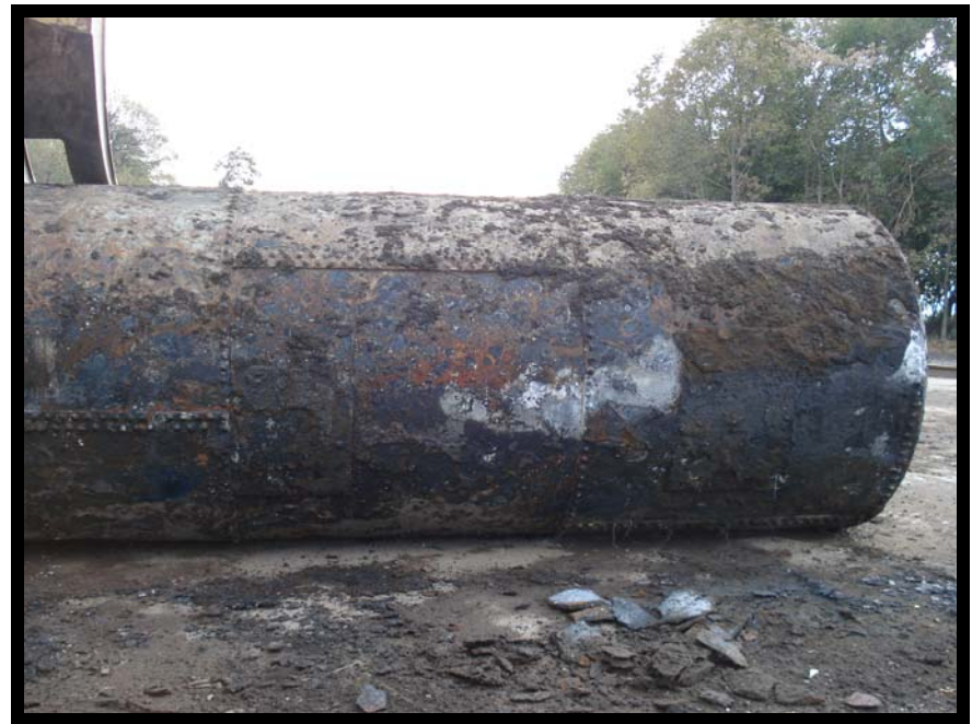
Photo 14 - View of UST B Bottom (North Side)
