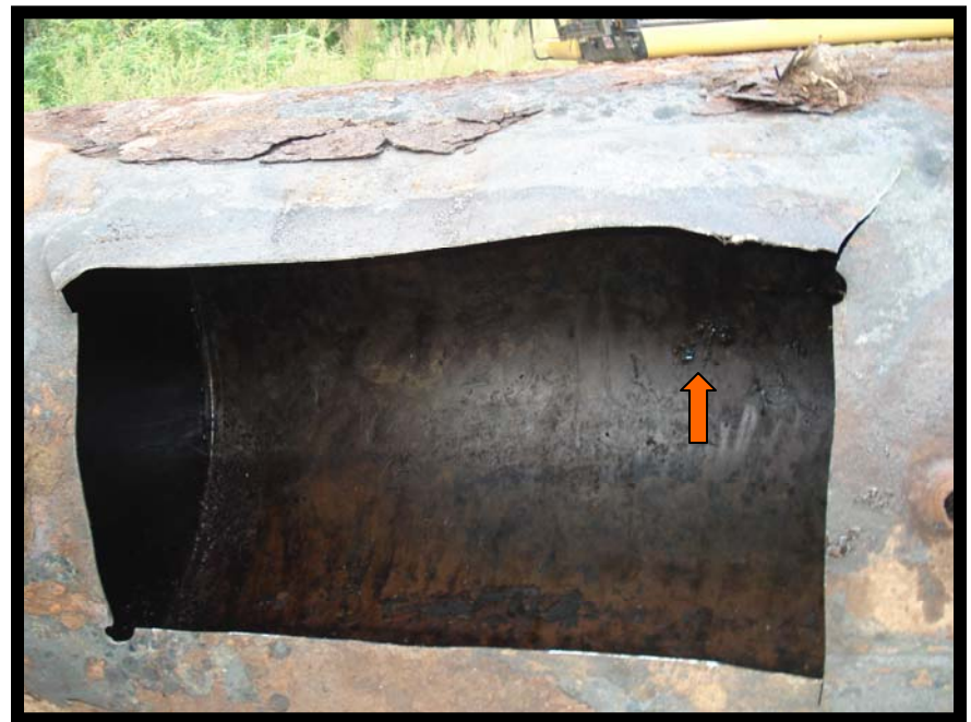
Photo 40- Hole Present in UST B after Scale Cleaning
