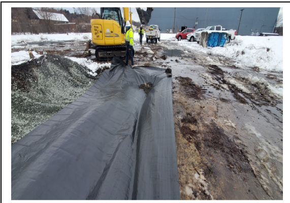
Fabric overlay of existing fabric and extended over concrete prior to placement of No. 2 Stone. Photo looking south.
