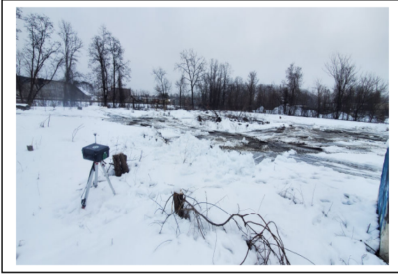
Looking northeast toward the breach area. Camp monitoring equipment in foreground left.
