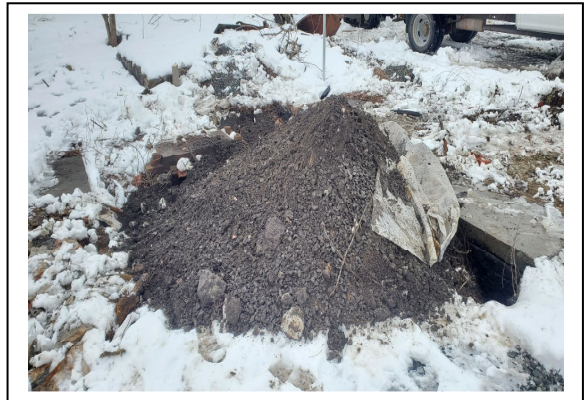
Flywheel area in which spoils from breach were placed prior to installing fabric over this area.
