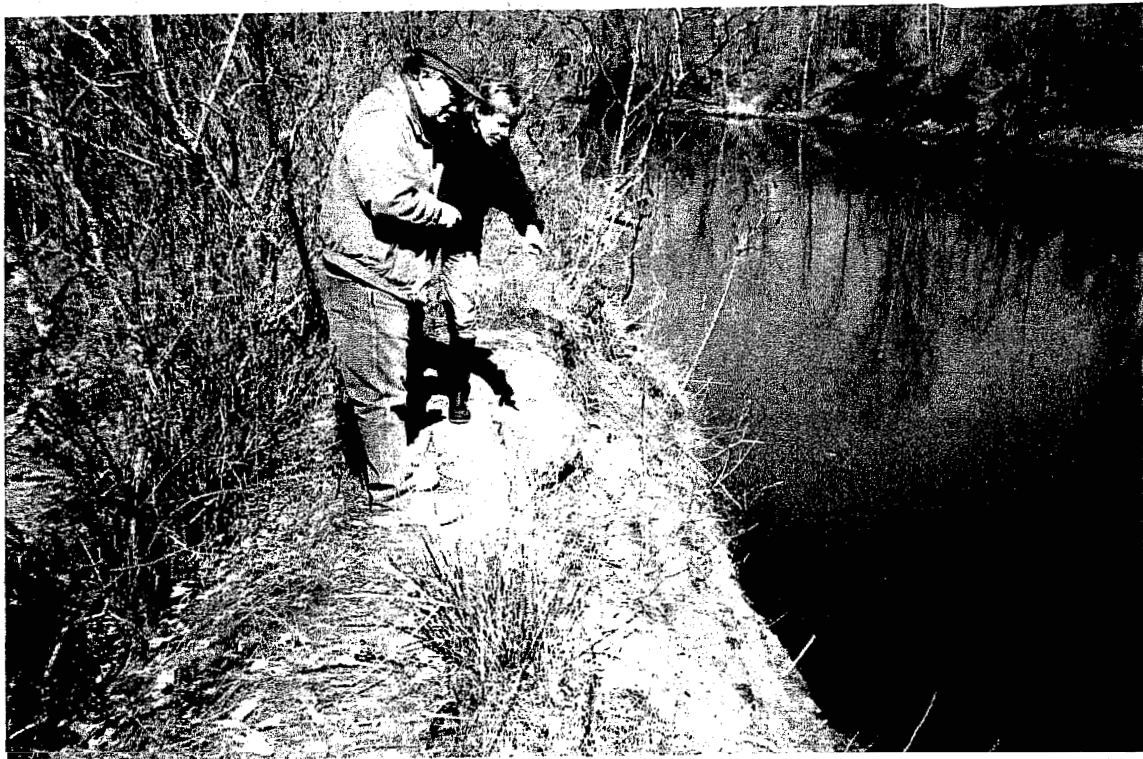
Willsboro Black Ash Site Top of Dike - Streambank Viewed West-Upstream. Note Black Discharge at Base of Slope
