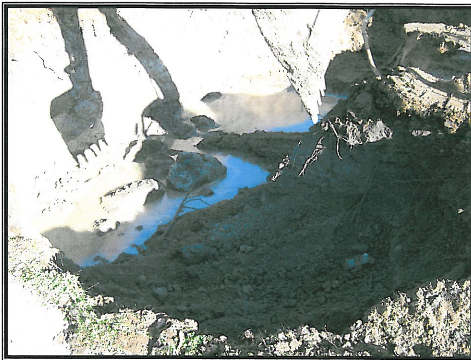
Photograph 2: Excavation Area Impacted By Damaged Water Line
