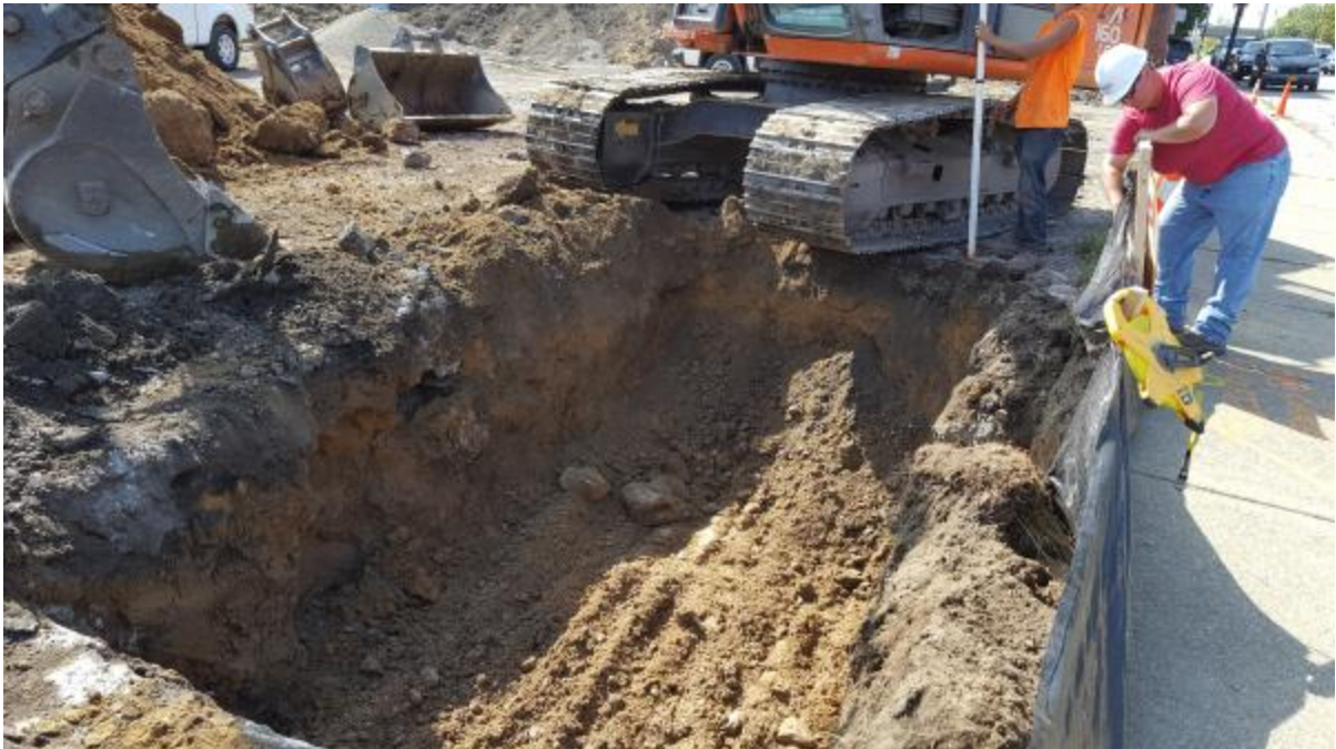
Photo 17 : Excavation of Area “C” – old wall encountered approximately 14 feet east of northwestern building corner of new building.
