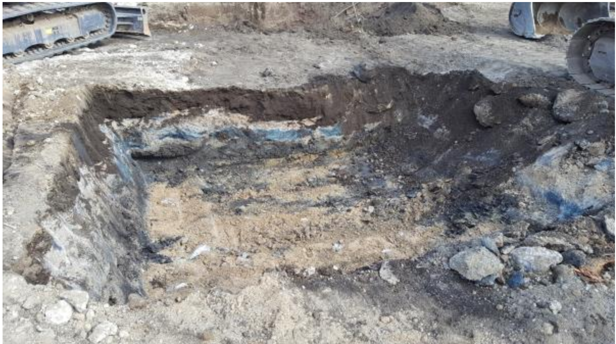
Photo 27 : Slag and debris fill at westernmost pier.
