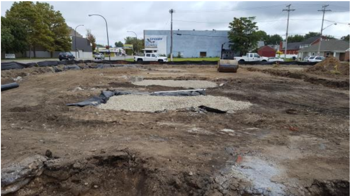
Photo 37 : Contractor placing fabric and stone in areas overexcavated due to fills and old concrete footings.
