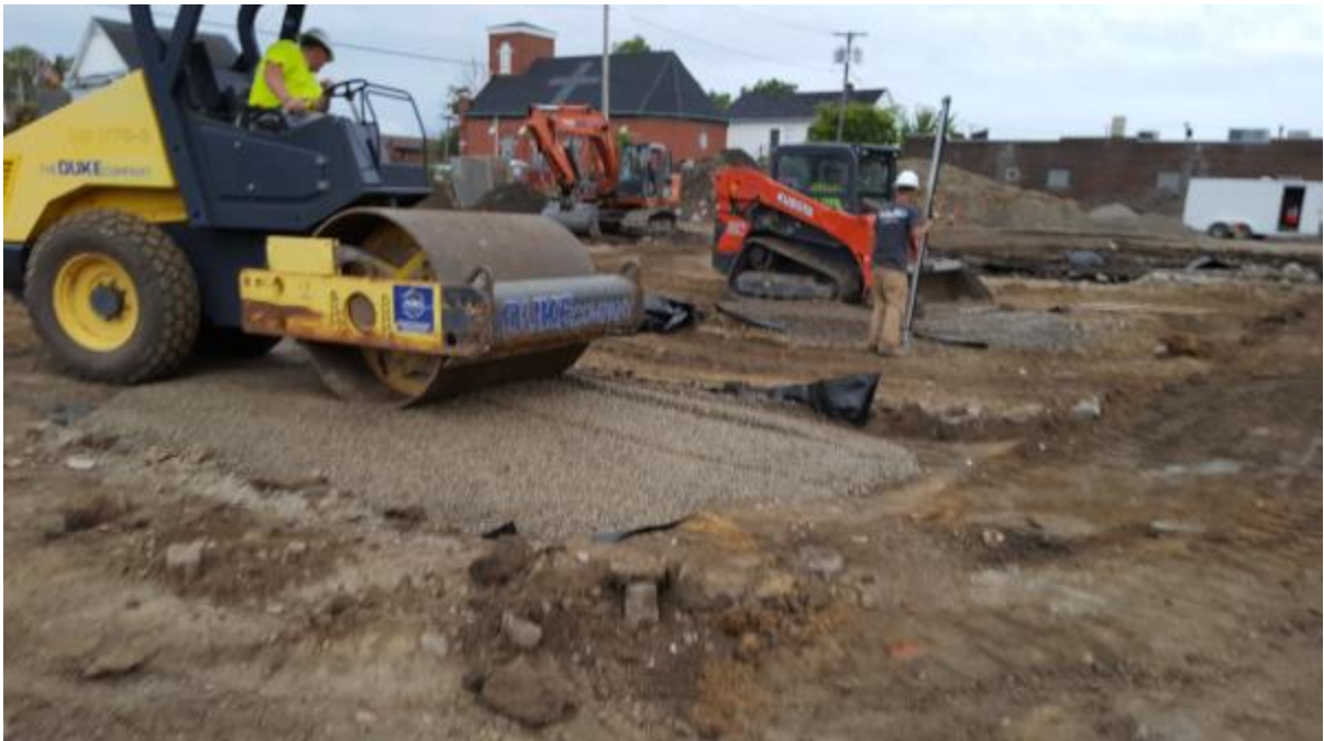
Photo 31 : View facing east from northwestern building corner – compacted stone to footing grade.
