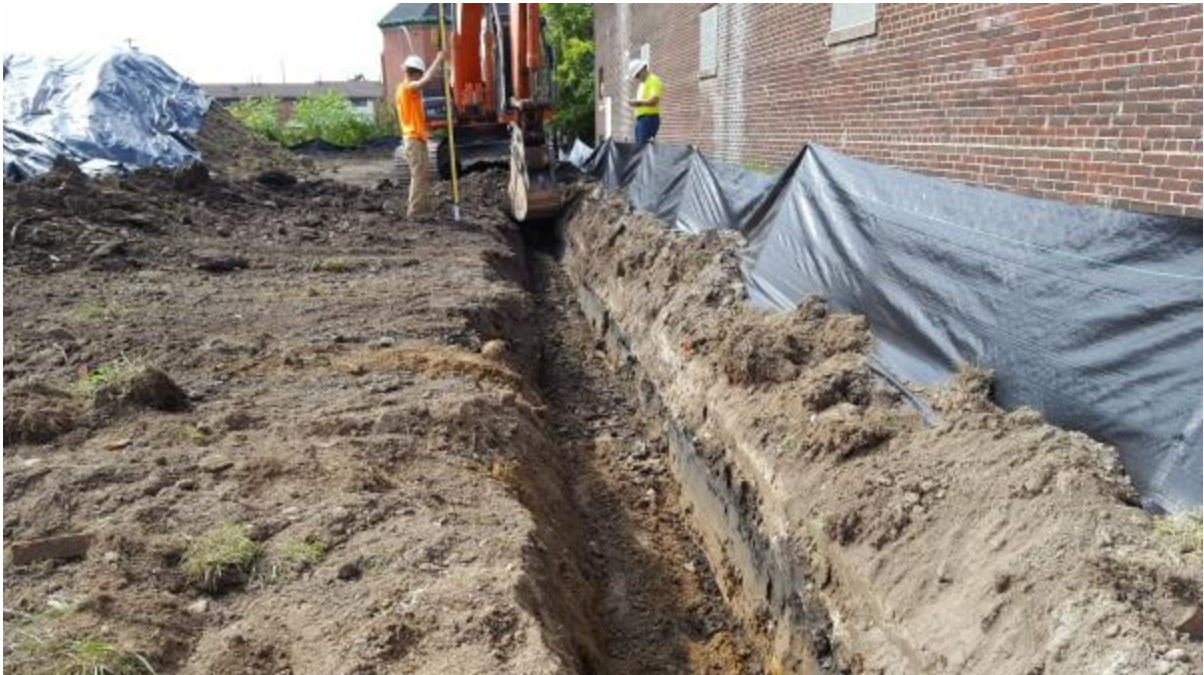
Photo 1 : Contractor preparing "Construction" entrance to site. Fills noted approximately 20' south of sidewalk off Ridge Road.
