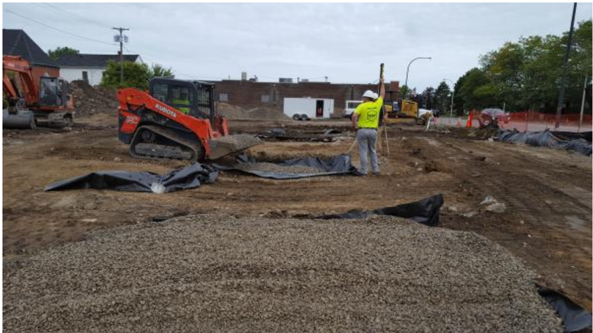
Photo 29 : Contractor compacting encapsulated stone fill placed at northeastern corner of building footing excavation.
