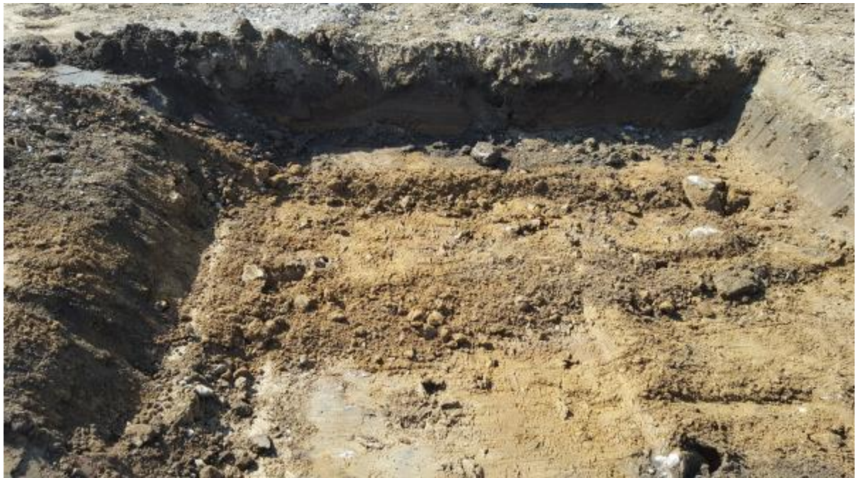
Photo 21 : Overexcavation at pier location due to organic and fills.
