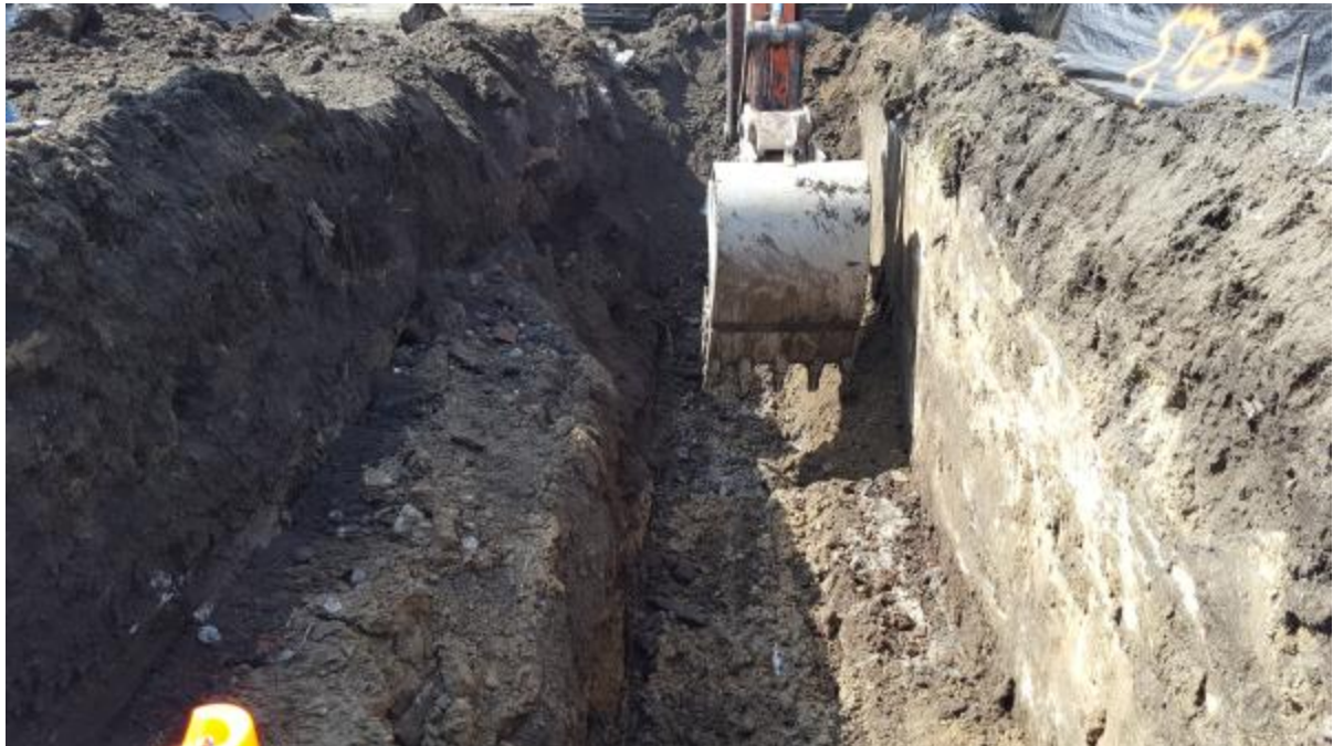
Photo 15 : Area "B" excavation – approximately 1.5 feet of fills underlain by firm native silty sands soils at bearing grade. Old footing wall encountered at end of trench by backhoe.
