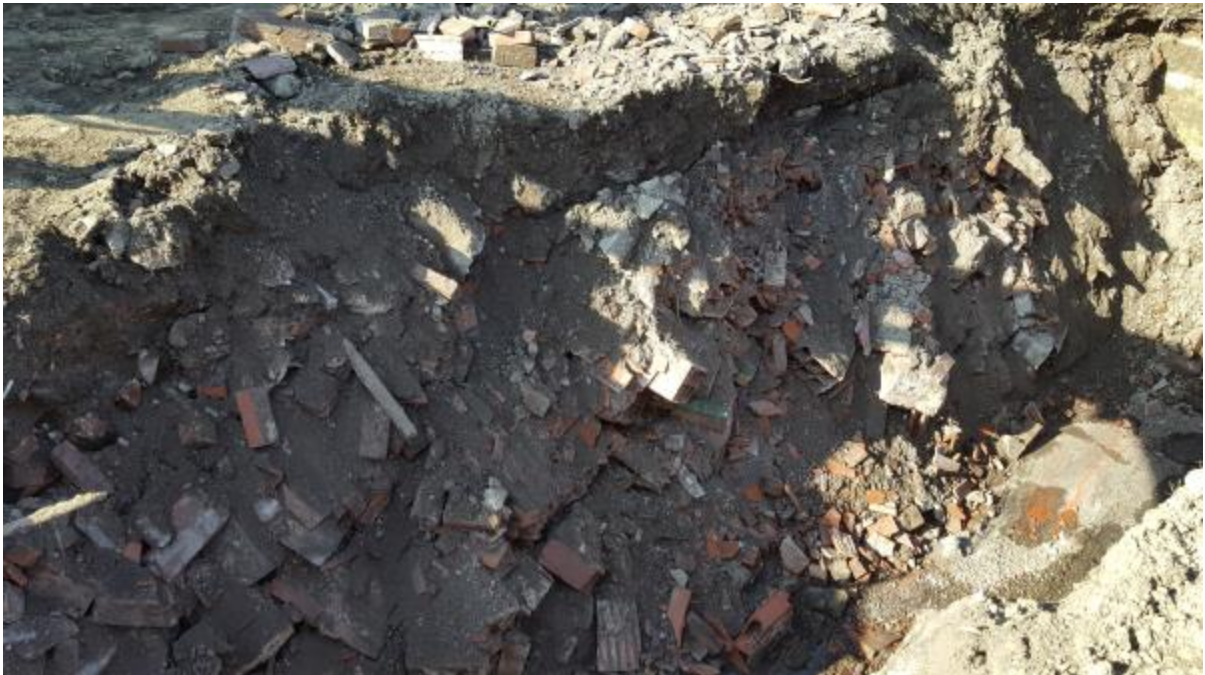
Photo 9 : Old basement wall encountered approximately 40' west of northeast building corner – Fill depth approximately 8.5 feet deep, with concrete slab at bottom.
