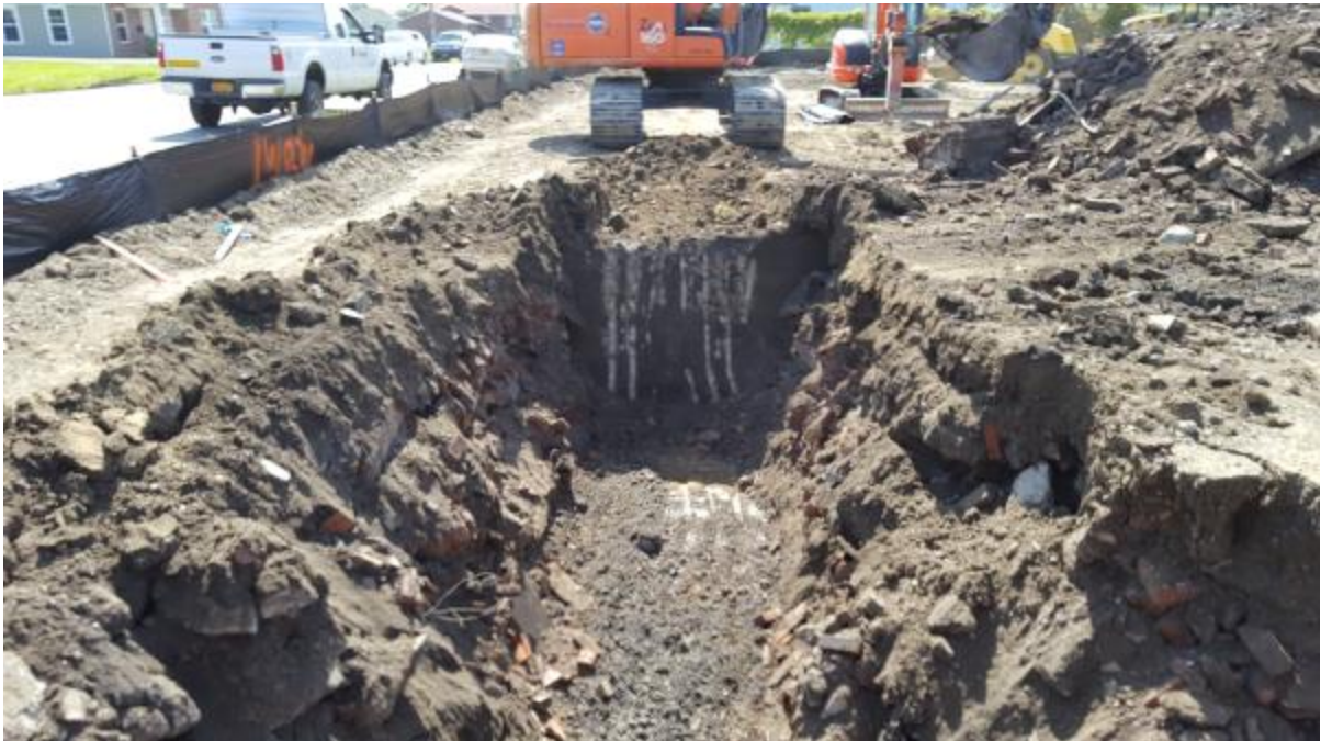
Photo 13 : Excavating south along eastern footing alignment of new building – from northeastern corner (Area “A”).
