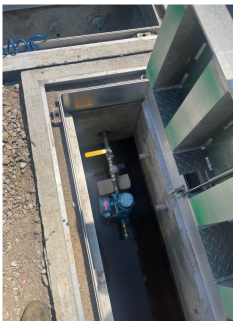
Photo 4: View facing north. View of installed product flow meter for RW-16R.
