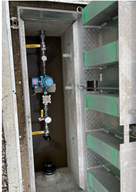
Photo 3: View facing east. View of piping in product metering vault.
