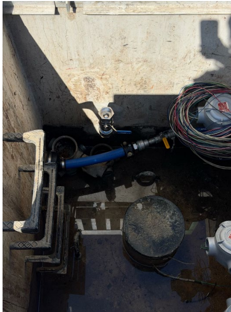
Photo 1: View facing south. Valve installed in RW-29R well vault.
