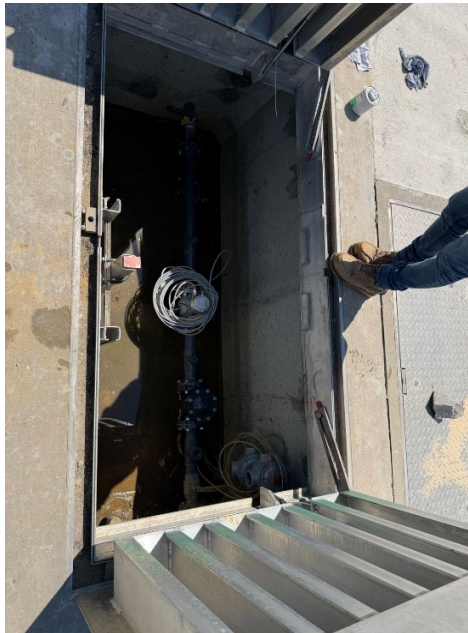
Photo 2: View facing south. PVC piping and flow meter installed in RW-29R water metering vault.
