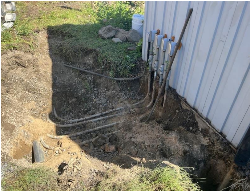
Photo 2: View facing south. Exposed conduit from wellhouse 14.
