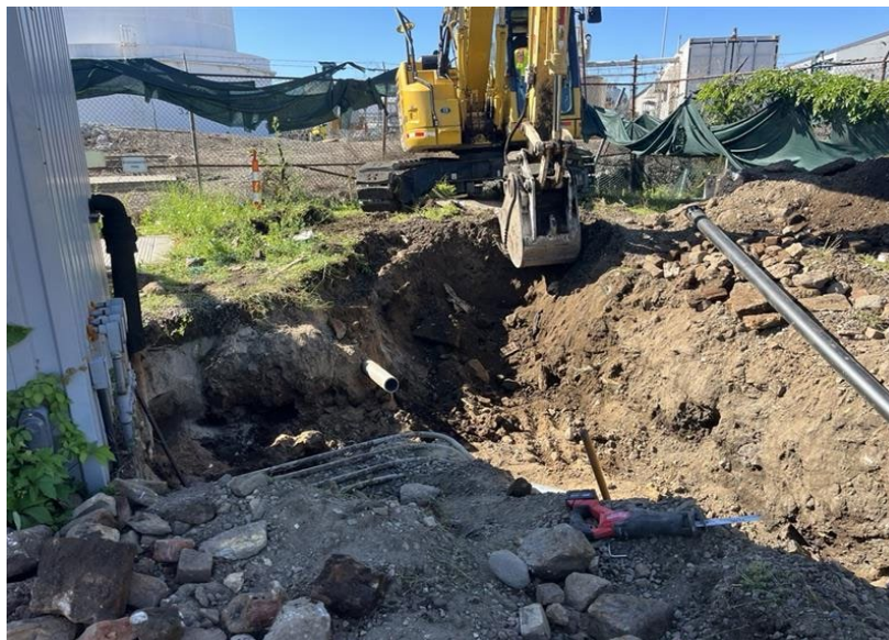
Photo 2: View facing south. View of exposed subsurface piping near wellhouse 14.
