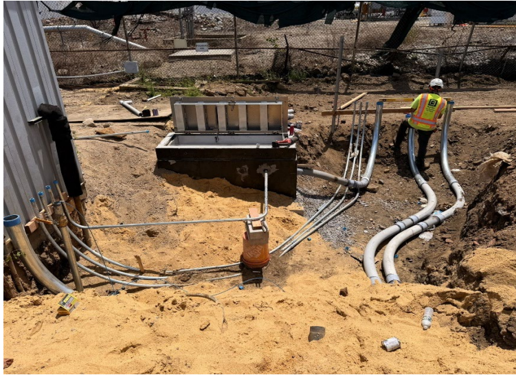
Photo 3: View facing south. View of piping for product storage tank and WH-14.
