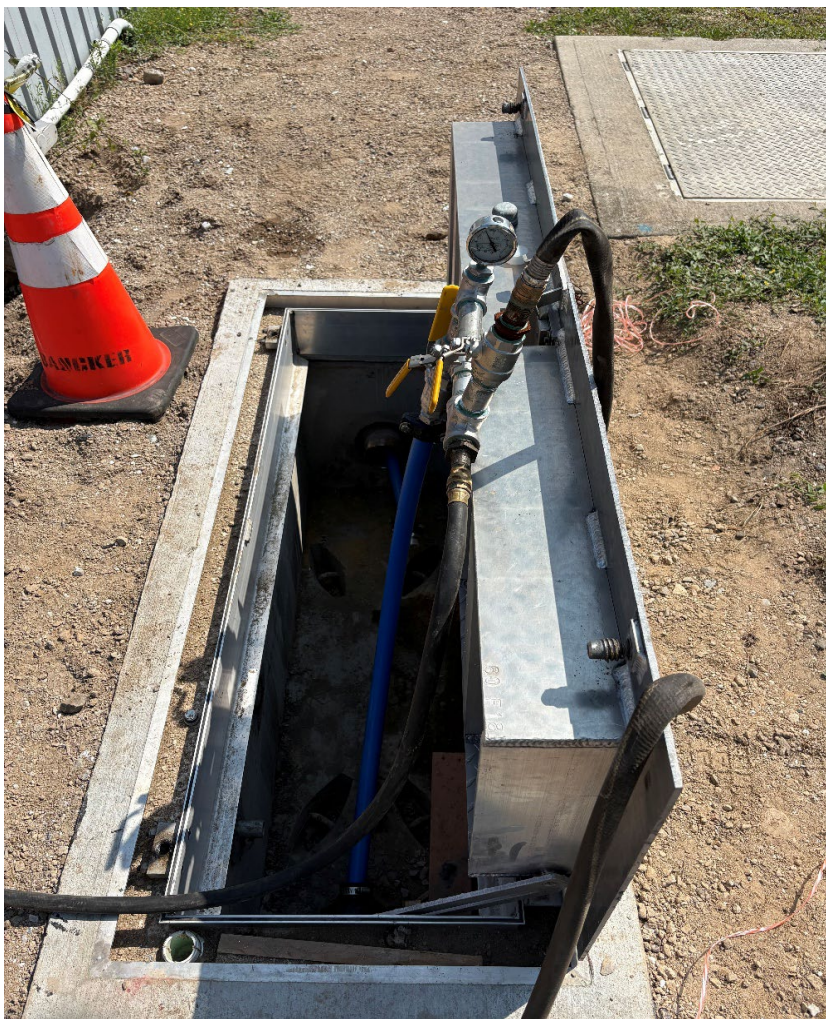
Photo 3: View facing east. Pressure test in product pull box.
