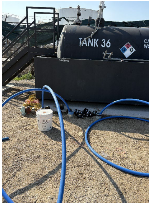
Photo 2: View facing south. View of product piping near relocated 2000 gallon tank.
