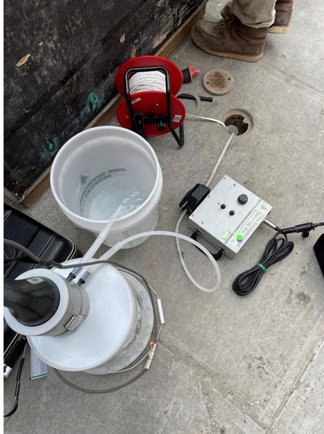
Photo 1: View of Langan purging monitoring well MW-4 along the 43 rd Avenue sidewalk (facing southwest).
