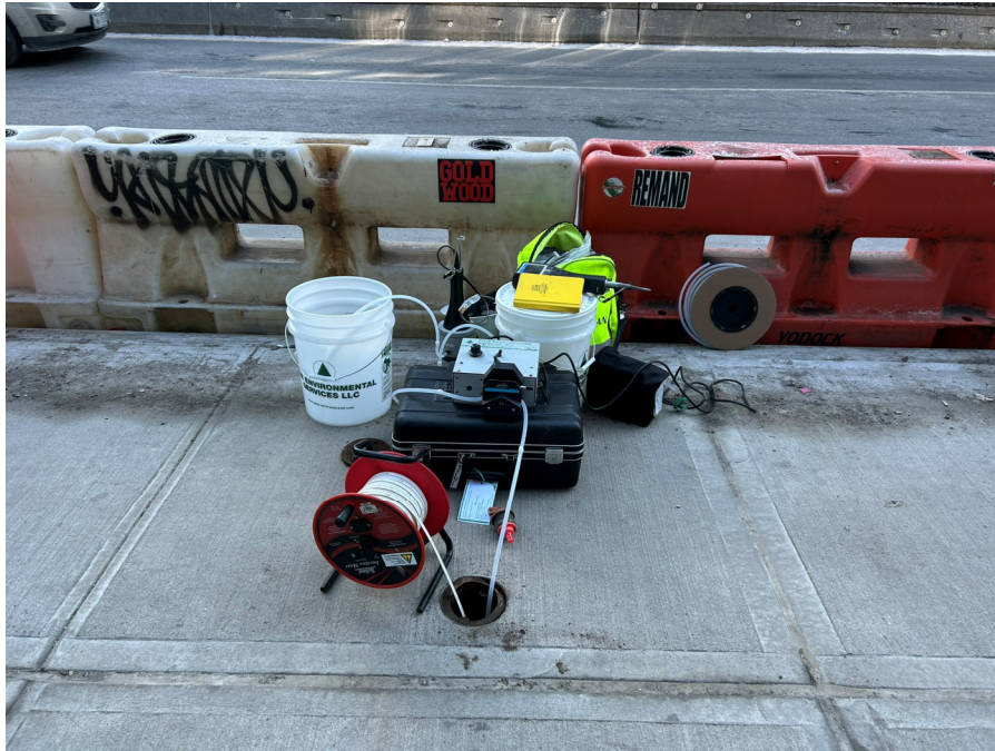
Photo 1: View of Langan purging monitoring well MW-1 along the Jackson Avenue sidewalk (facing south).
