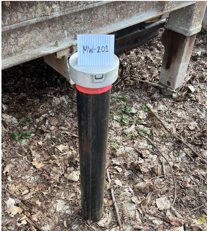
Photograph No. 11: MW-201 Pre abandonment 04/11/2023
