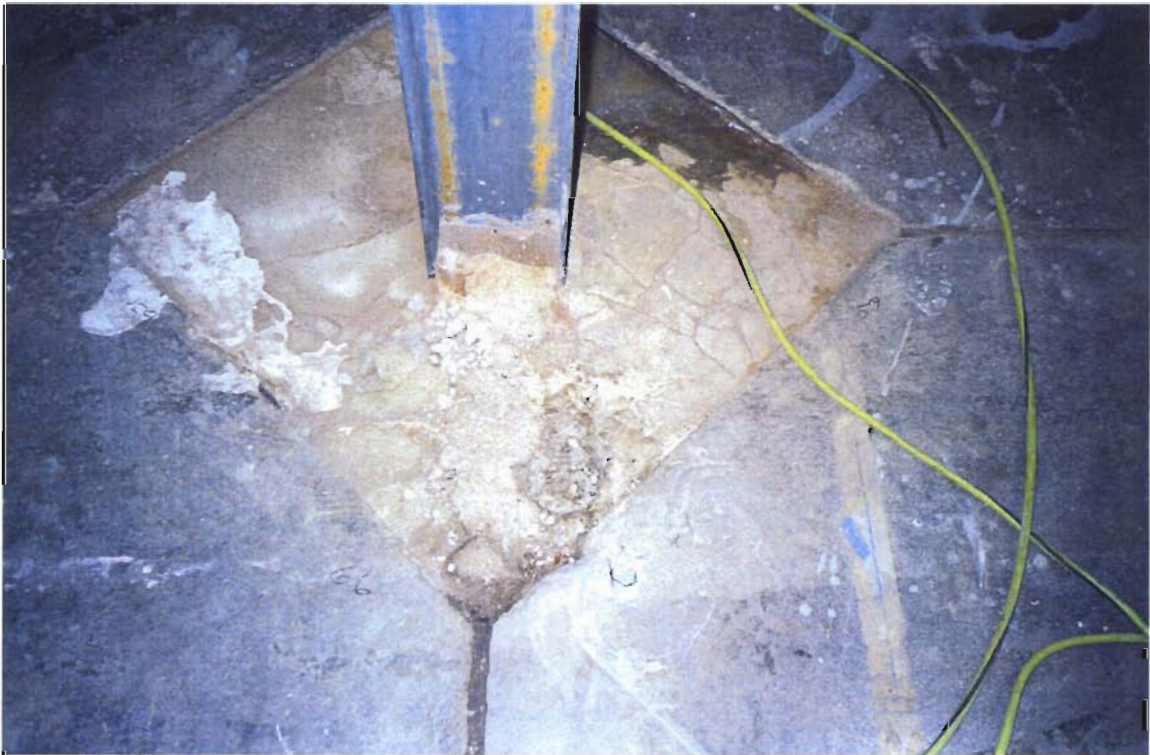
Pole with radiation in concrete. Area was bored and no radiation was detected.
