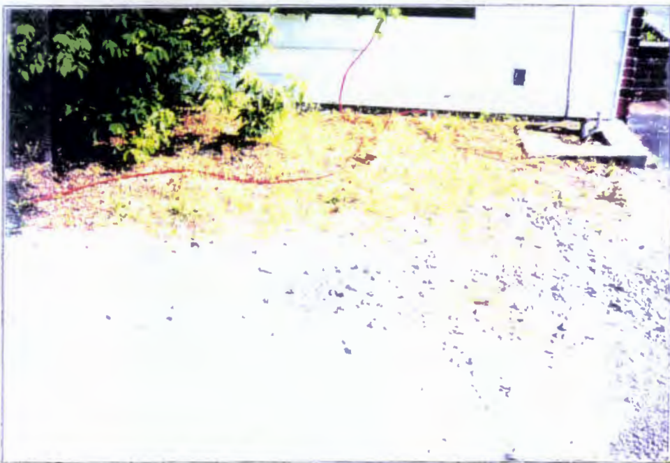
Fill ports for tanks along south edge of building structure
