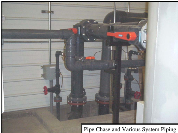
Pipe Chase and Various System Piping
