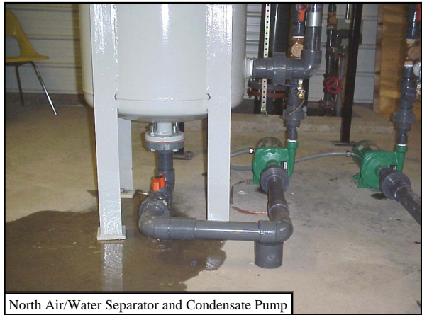
North Air/Water Separator and Condensate Pump
