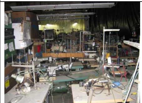
Photo 9 is a typical view of mitigation area 3 showing stored materials which need to be moved prior to ASD install.
