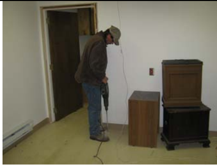
Photo 2 is a typical view of an installation of a vacuum diagnostic test hole.
