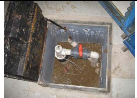
Photo 6 shows an existing exterior point sump pit that needs sealing.
