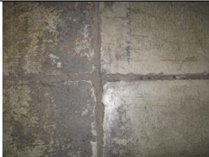
Photo 5 shows typical floor slab expansion joints which need sealing.
