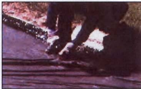
Photograph of wrinkle that requires repair.
