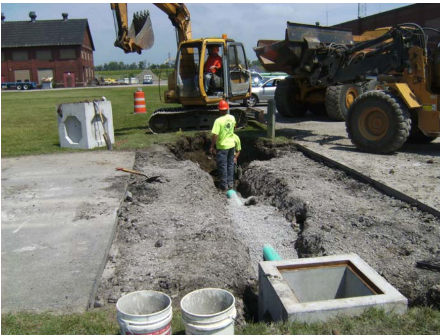
June 26, 2008 Installation of 6" HDPE piping between two catch basins north of installed Building 8 Asphalt Cap.
