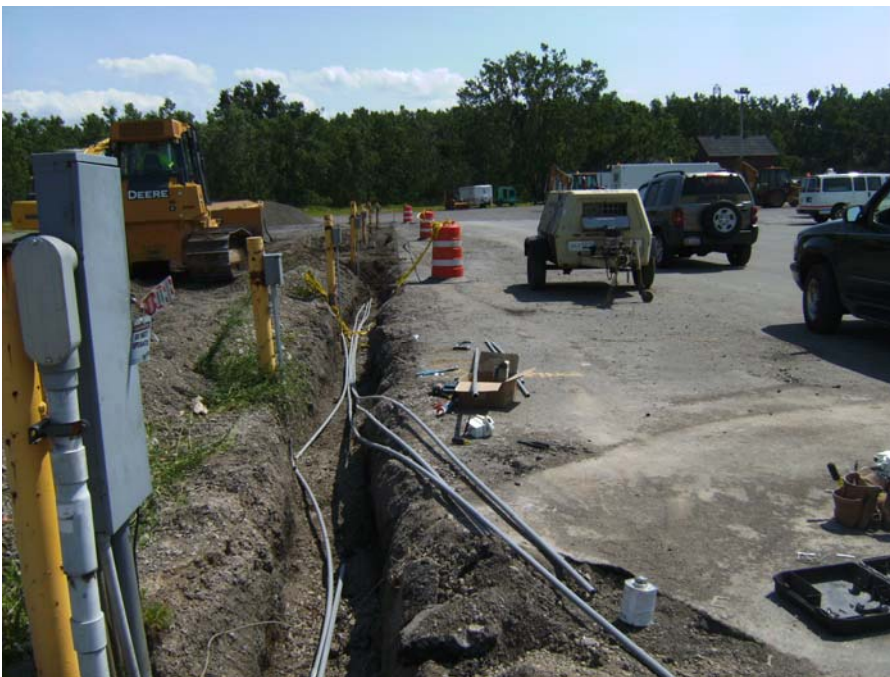
July 7, 2008 Installation of electrical conduit along western edge of installed Building 8 Asphalt Cap.
