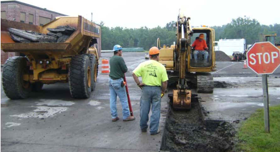
June 27, 2008 Trenching for installation of catch basin north of installed Building 8 Asphalt Cap.
