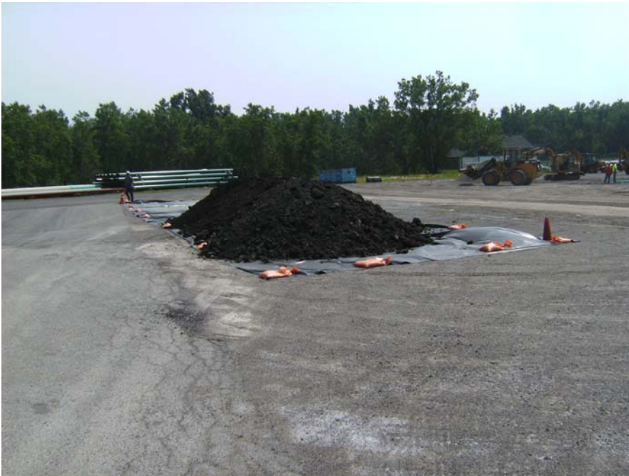
June 30, 2008 Contaminated soil staging east of installed Building 8 Asphalt Cap (south of Building 8).
