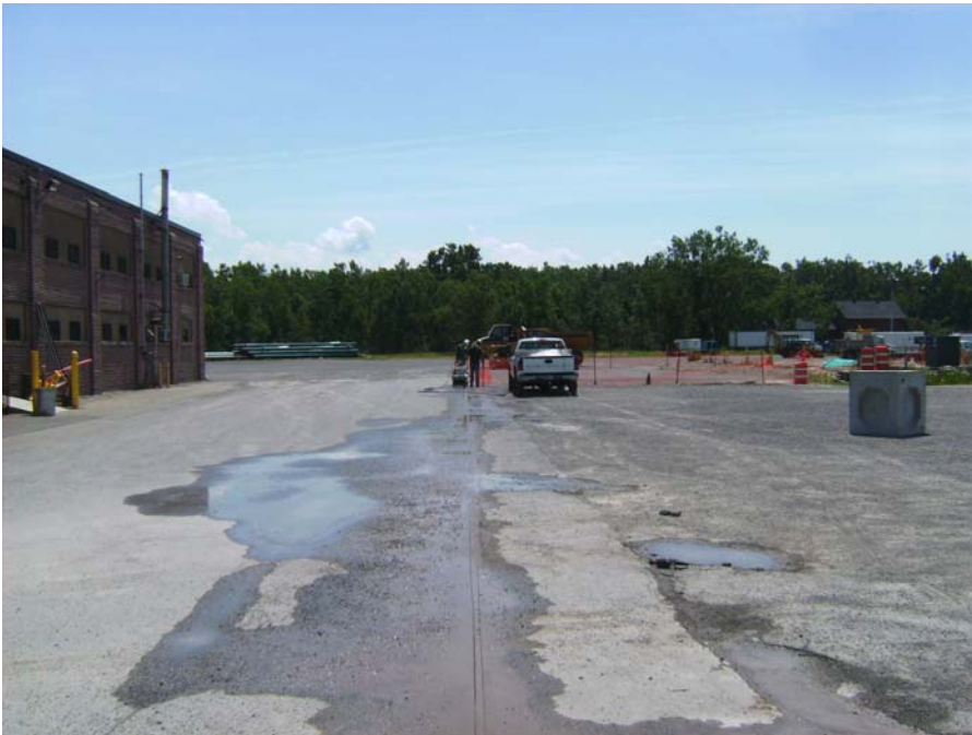
June 25, 2008 Saw cutting of existing pavement with water spray to control dust generation.
