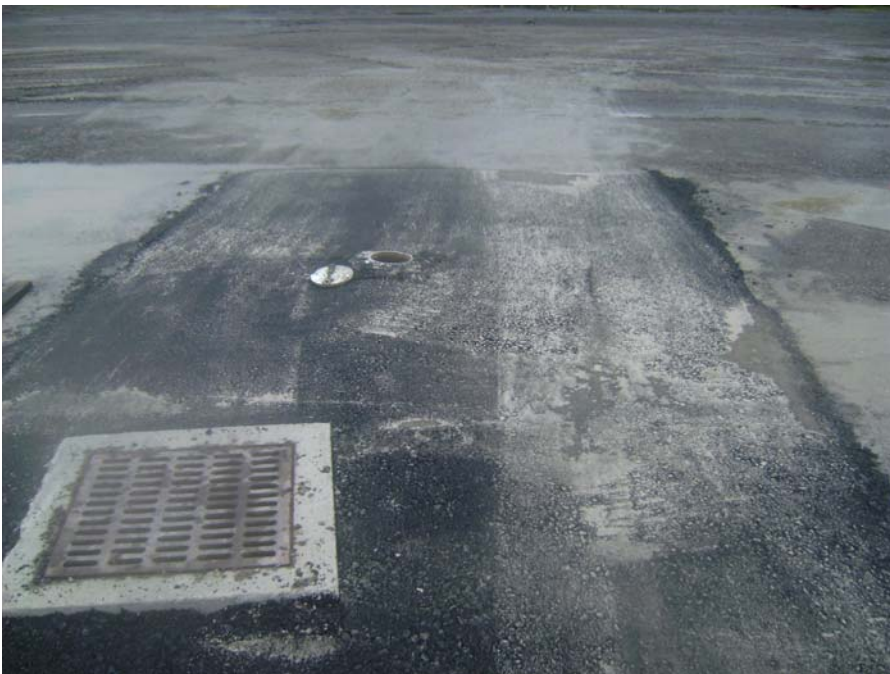
July 9, 2008 Existing catch basin and monitoring well MW-7 following installation of asphalt binder material.
