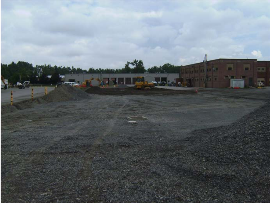
June 30, 2008 Rough grading and compaction of surface material and borrow source material.
