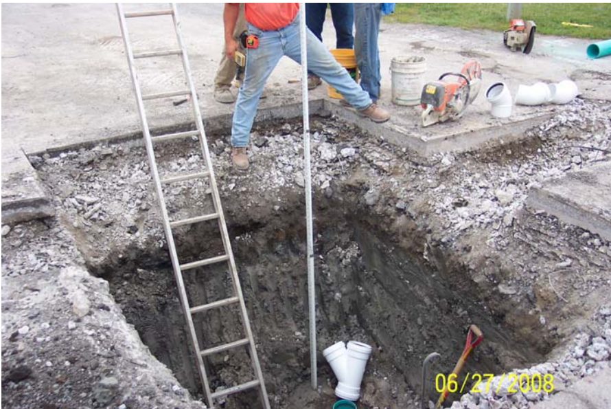
June 27, 2008 Preparation of the 36" sewer for the 6" drain connection north of installed Building 8 Asphalt Cap.
