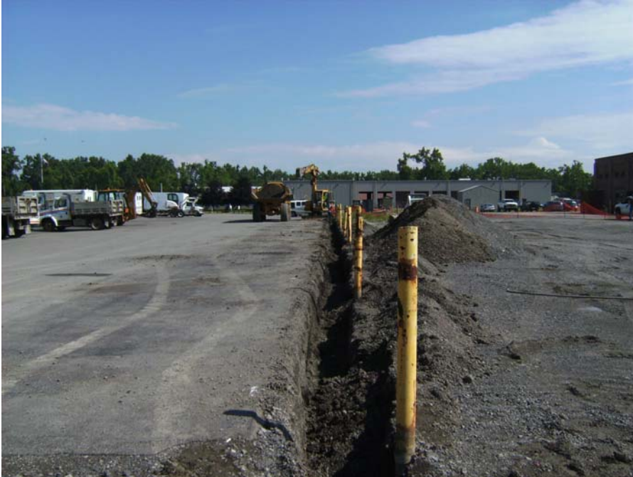
June 30, 2008 Trenching for installation of electrical conduit along western edge of installed Building 8 Asphalt Cap.
