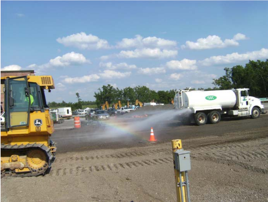
July 8, 2008 Water spray to control dust generation and aid in the compaction of the Building 8 Asphalt Cap.
