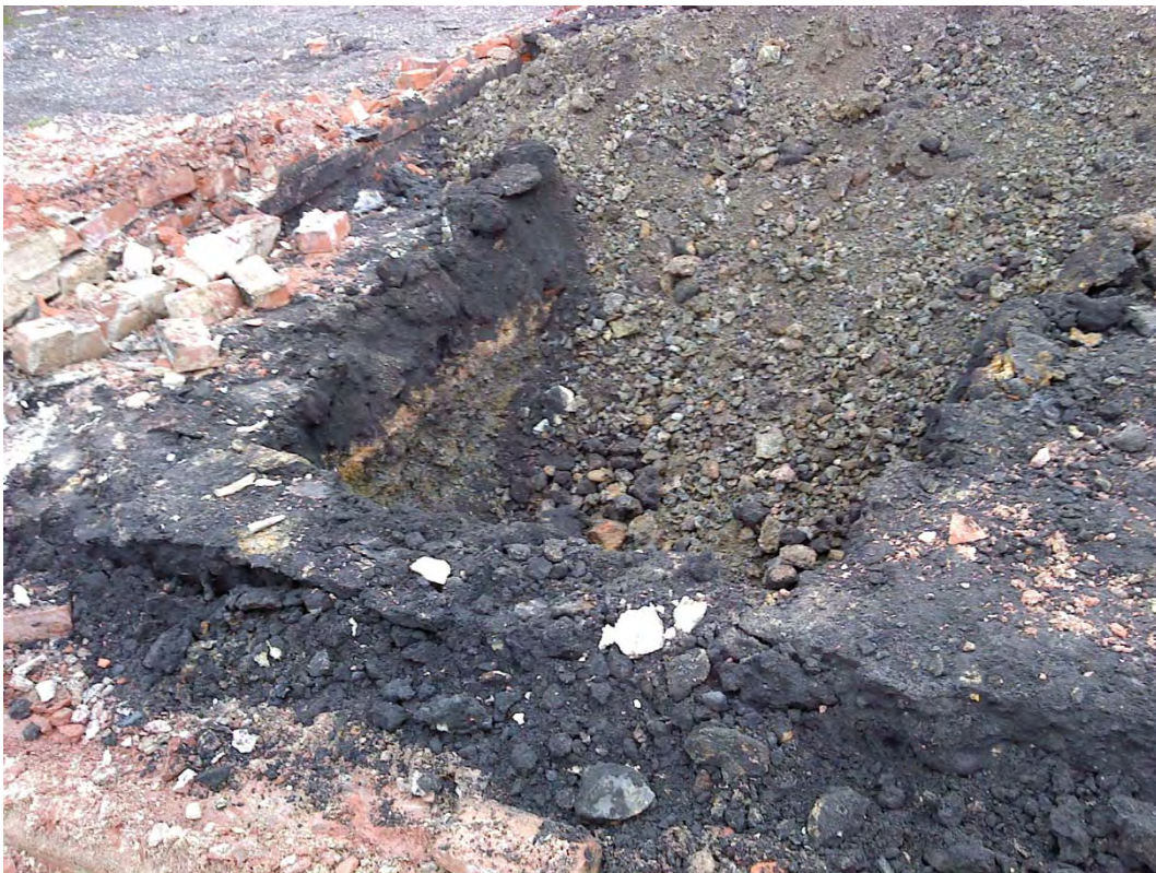
Coal slag material used for bedding was exposed after removing the concrete floor surface.
