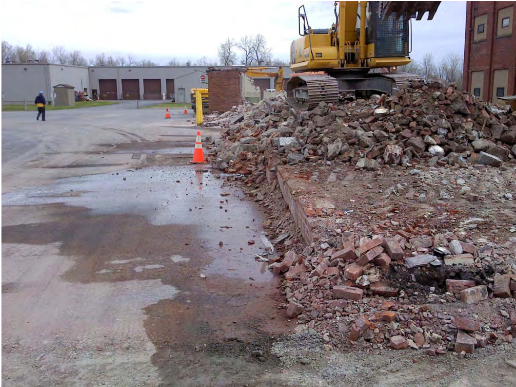
The concrete floor surface became exposed as debris was prepared for loading out.
