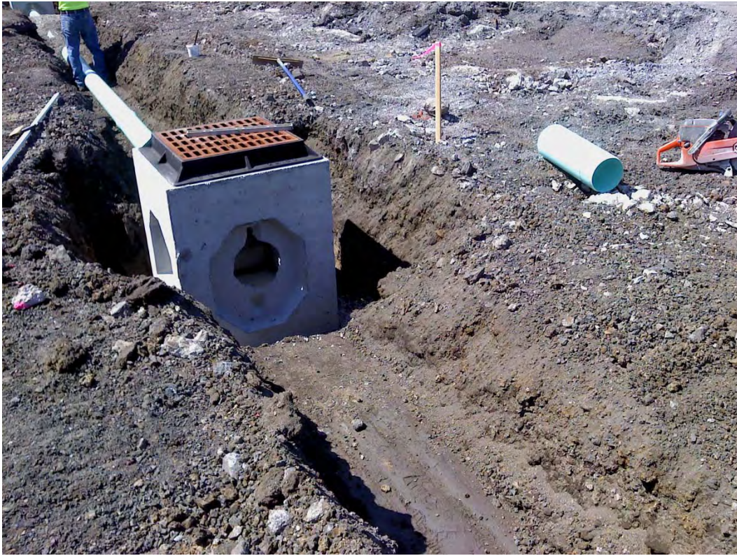
Second storm water catch basin.
