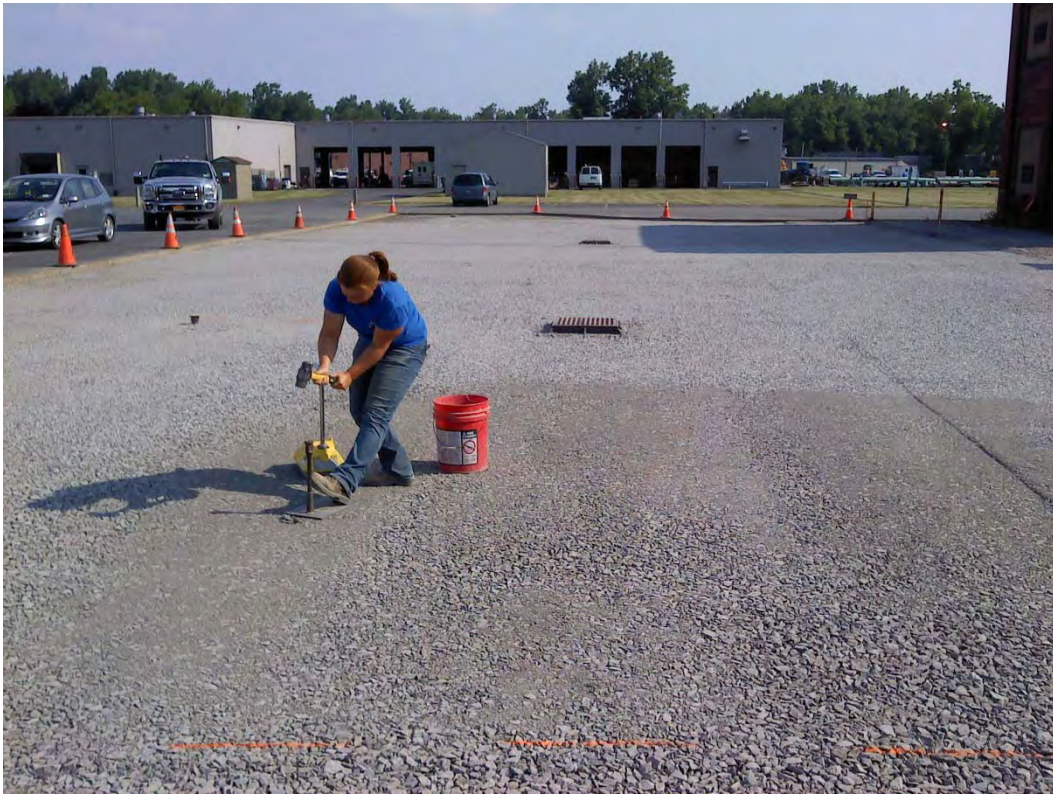
Technician conducting Proctor Test to check compaction of new crushed stone sub base.
