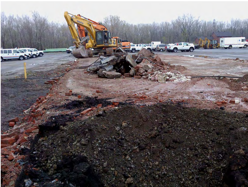
Concrete floor debris piled on top of floor bedding.
